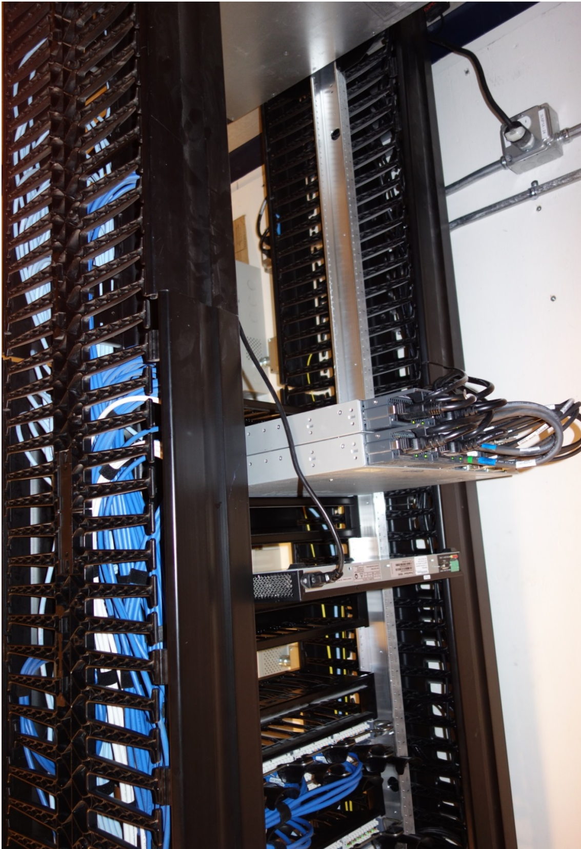
Permission obtained for this rack in a small room – back view.
