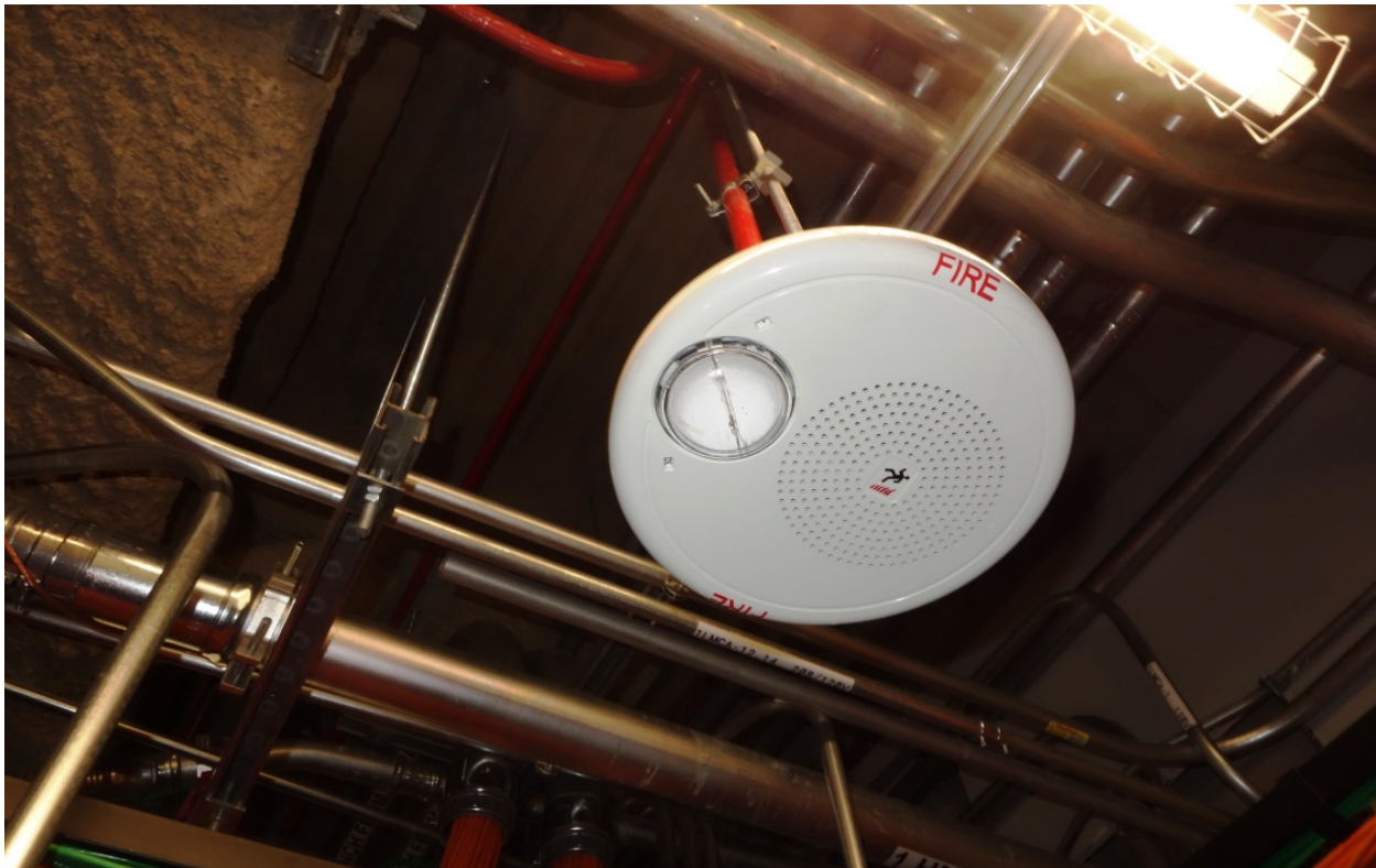
Sample IT Room smoke detector.
