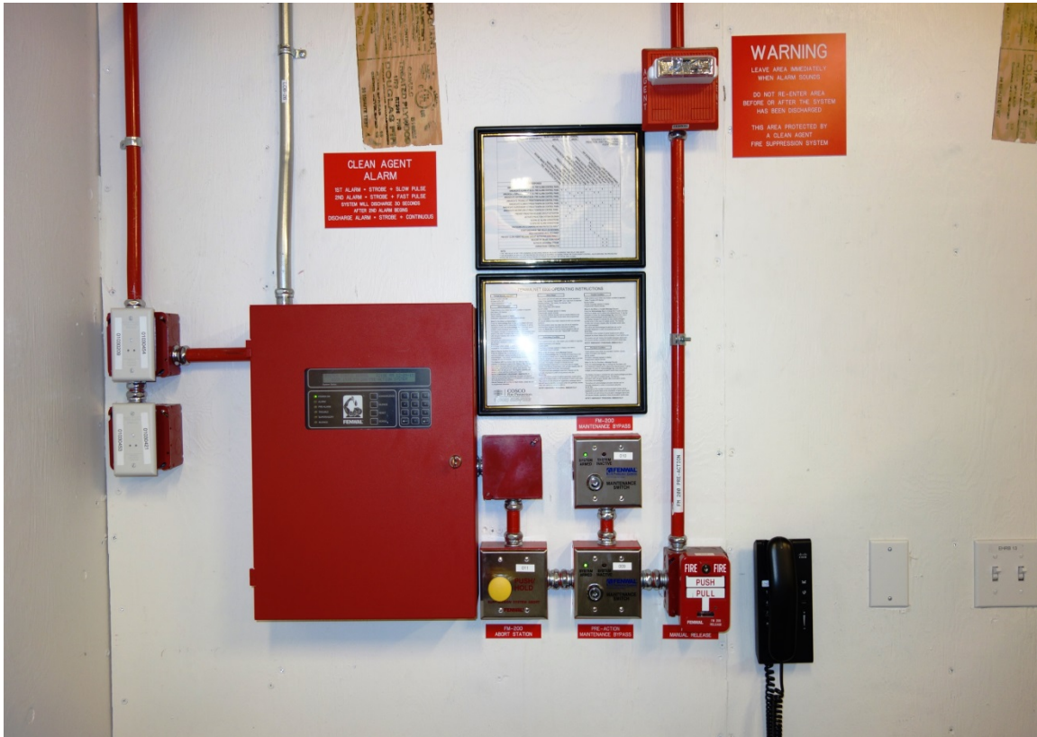
Sample fire alarm annunciator panel.
