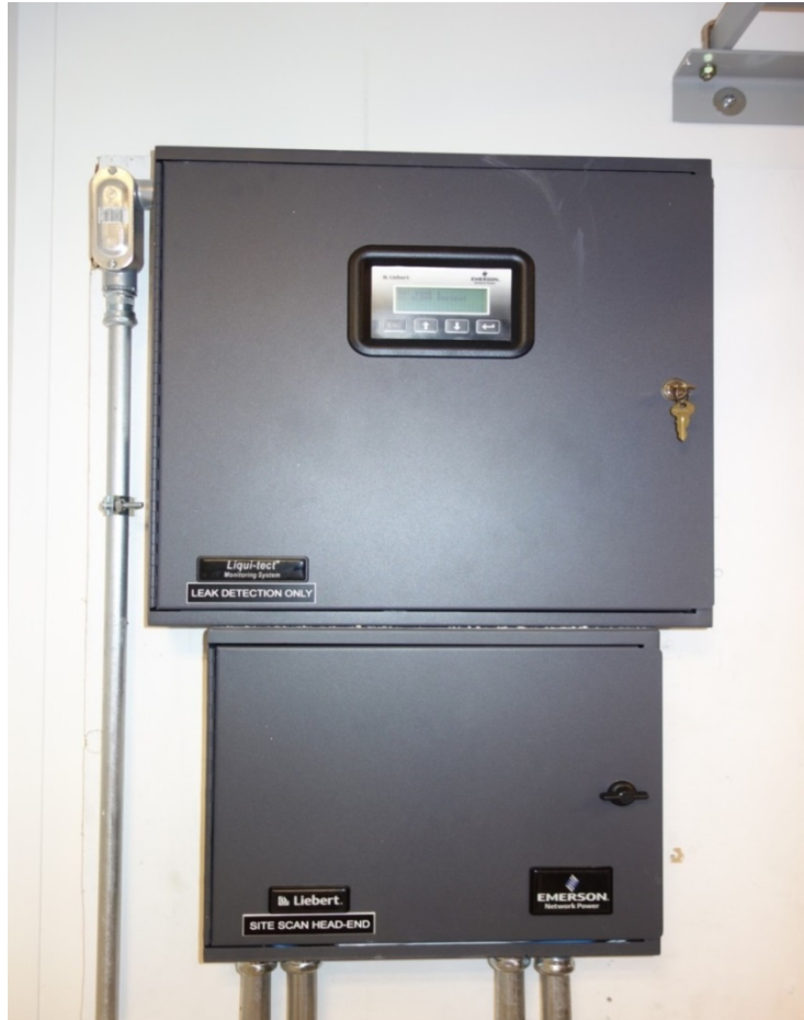
Liebert Site Scan electrical/mechanical monitoring units.
