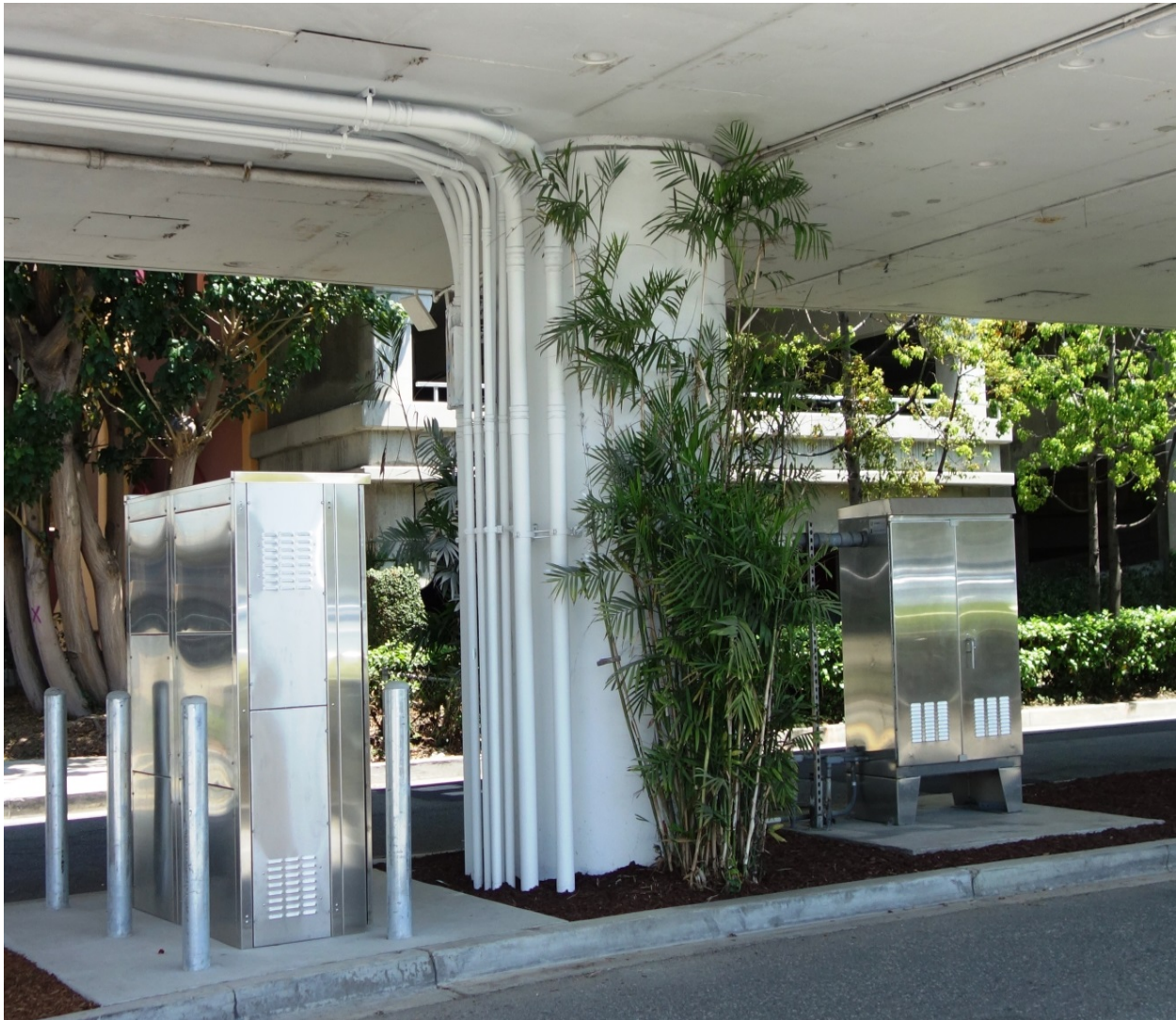
Outdoor TE's with vents for ambient air cooling.
