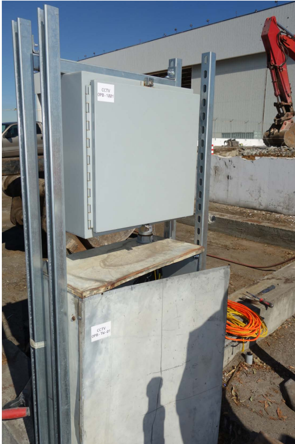
Steel NEMA 4 TE's are permitted for temporary jobs up to 12-months duration.
