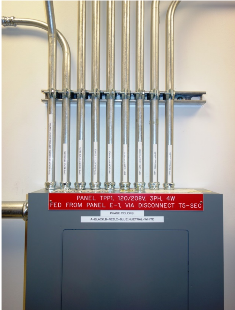
Electric panel and conduits shall be labeled per the LAWA D&CH.
