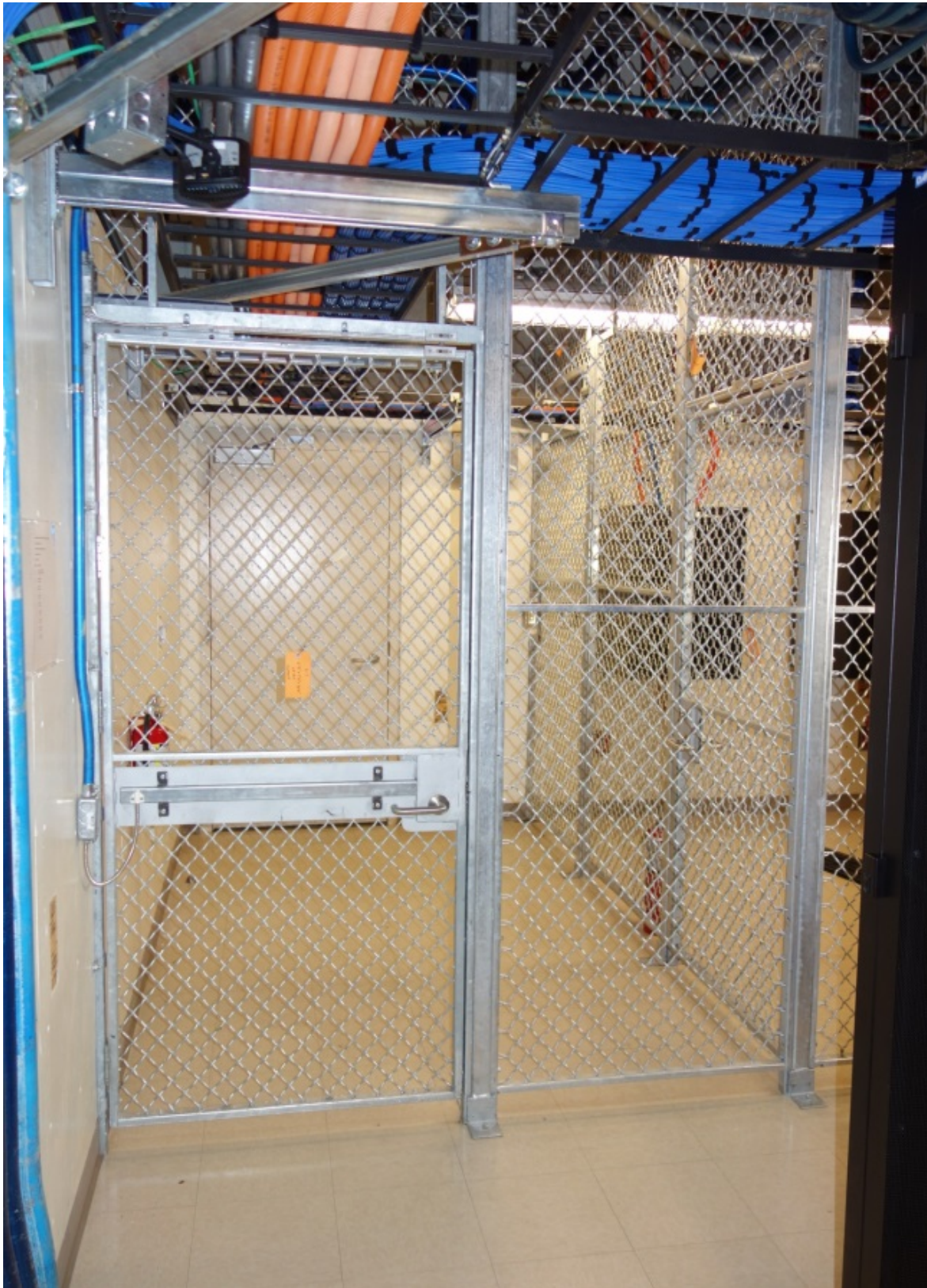
Chain link divider separating TCWC adjacent to an IT Room. Camera is the facing entrance foyer.
