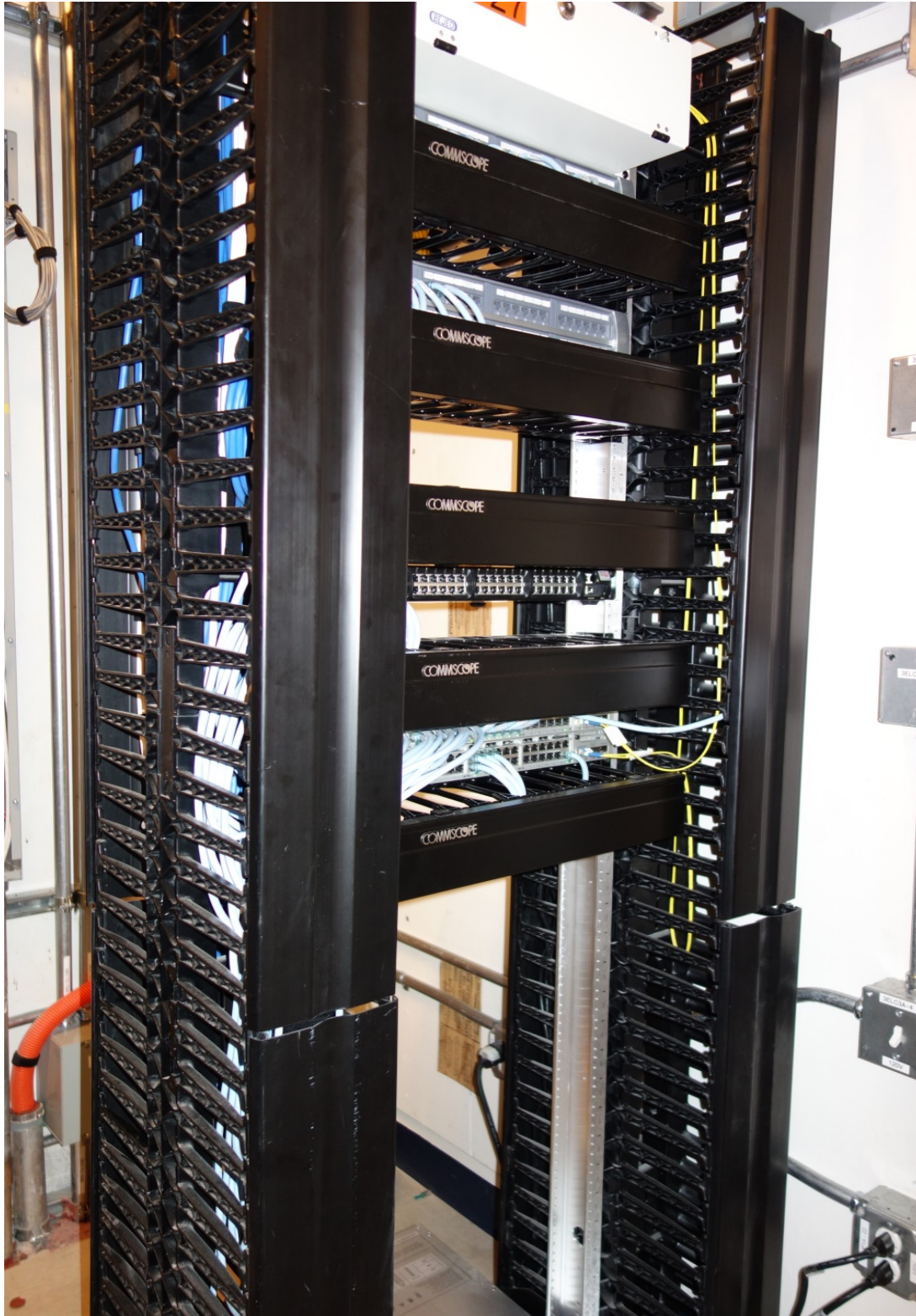
Permission obtained for this rack in a small room – front view.
