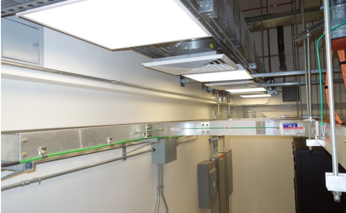
2' x 2' LED light fixtures.
