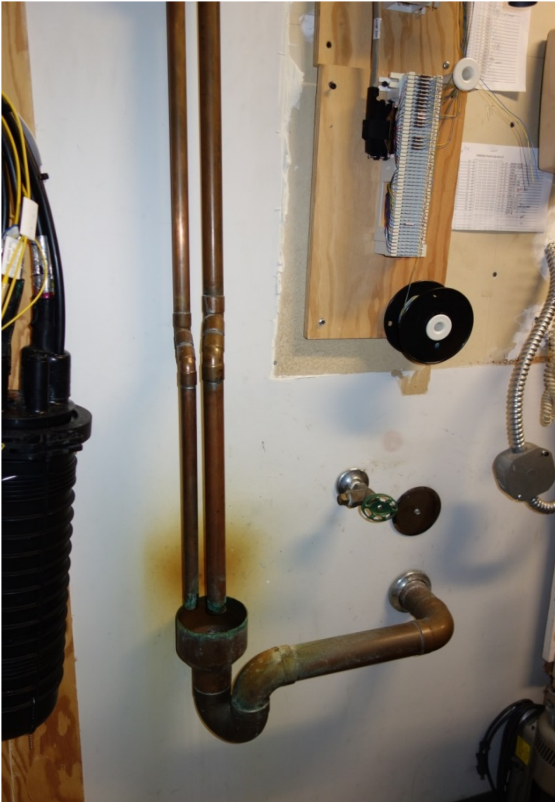
Legacy HVAC condensate wall drain.
