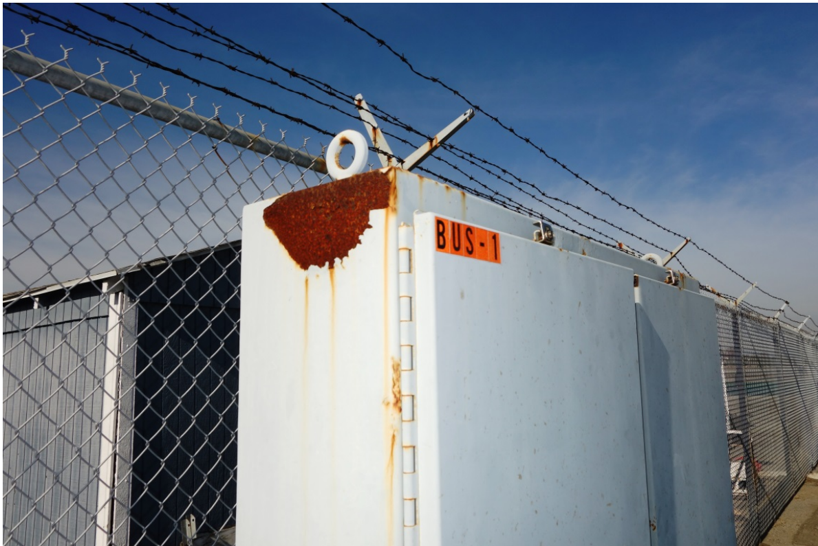
A legacy outdoor TE with appropriate labeling. Rust is the reason for switching to Stainless Steel.
