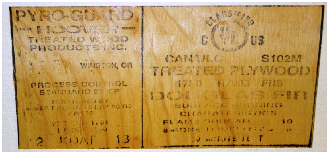
Unpainted stamps for local AHJ inspection.
