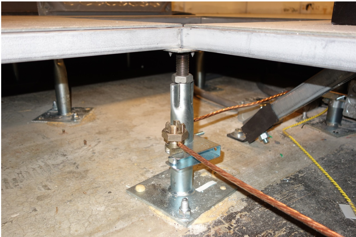
Grounding is required on raised access floors.
