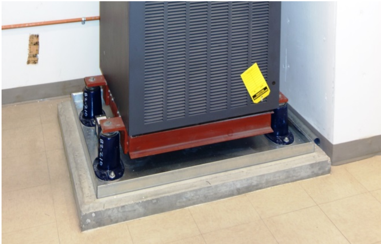
Enlargement of the condensate HVAC drip pan.
