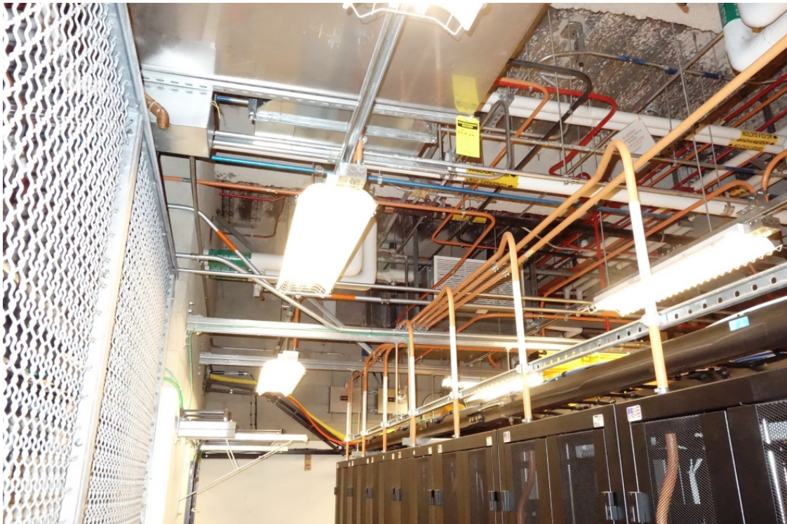
4-foot LED light fixtures.
