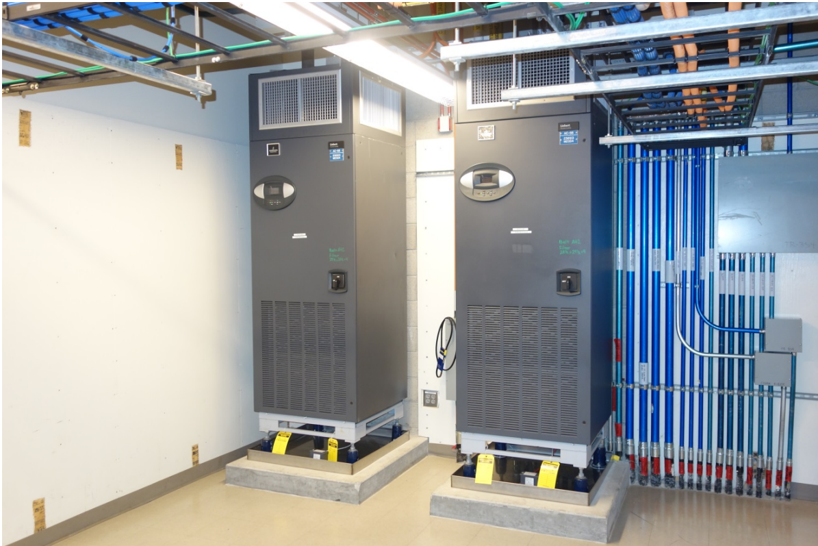
HVAC condensate containment pans prevent wet IT Room floors.
