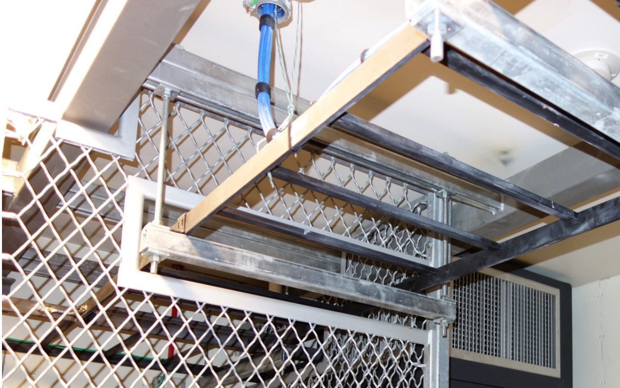
Divider wall enclosing ladder rack.
