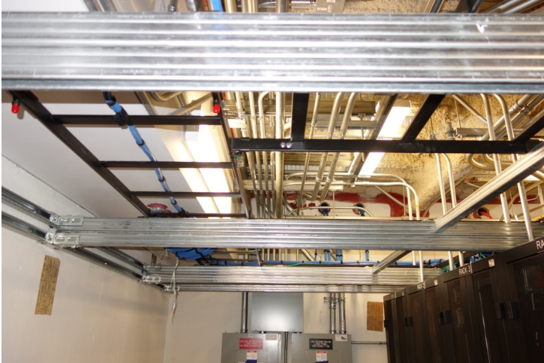
A strut framework for the seismic anchoring of cabinets ladder rack is shown.
