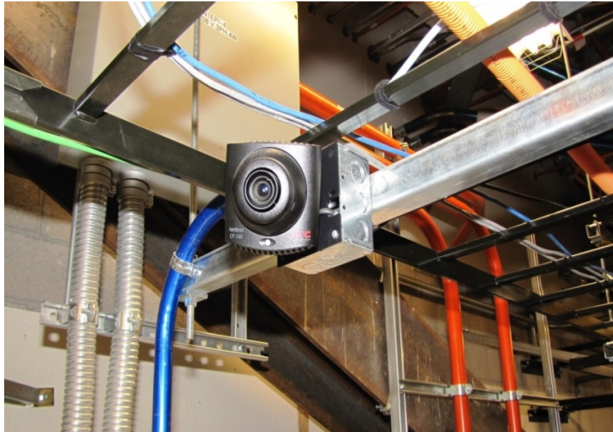
Sample Legacy Netbotz surveillance camera - No longer used in IT rooms.
