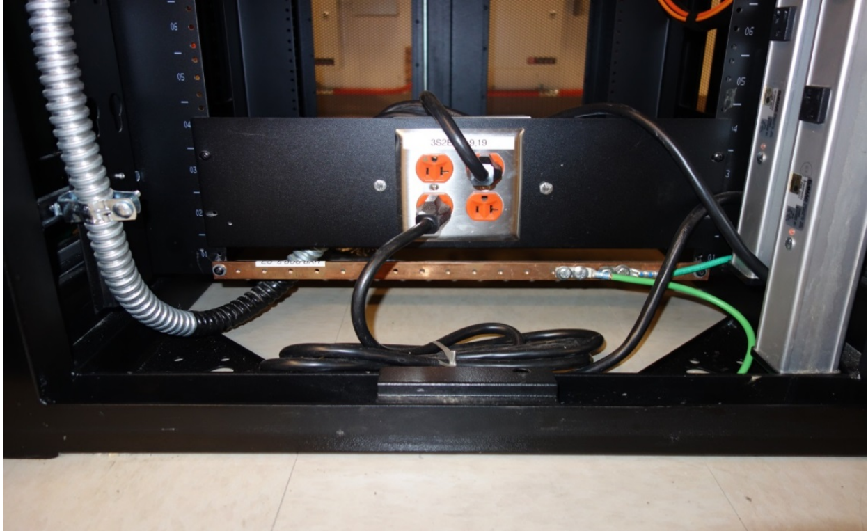
Standard equipment cabinet equipment grounding bus bar shown.
