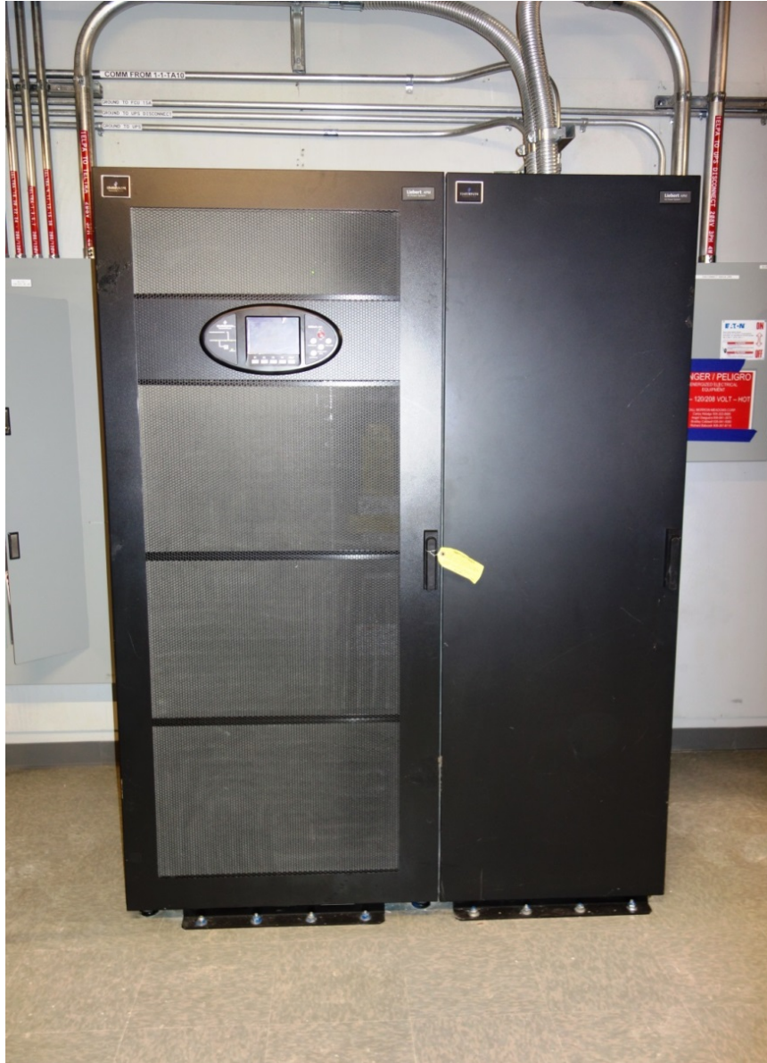
A 20 kVA Liebert UPS and battery cabinet shown.
