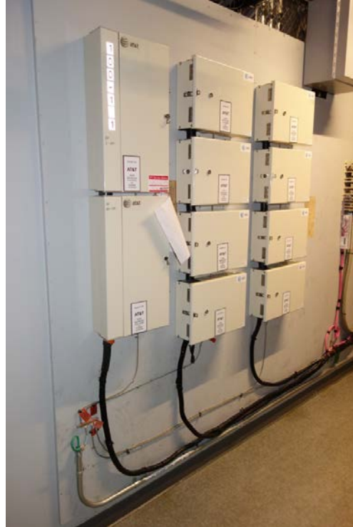
Mid-sized Copper Entrance Facility.
