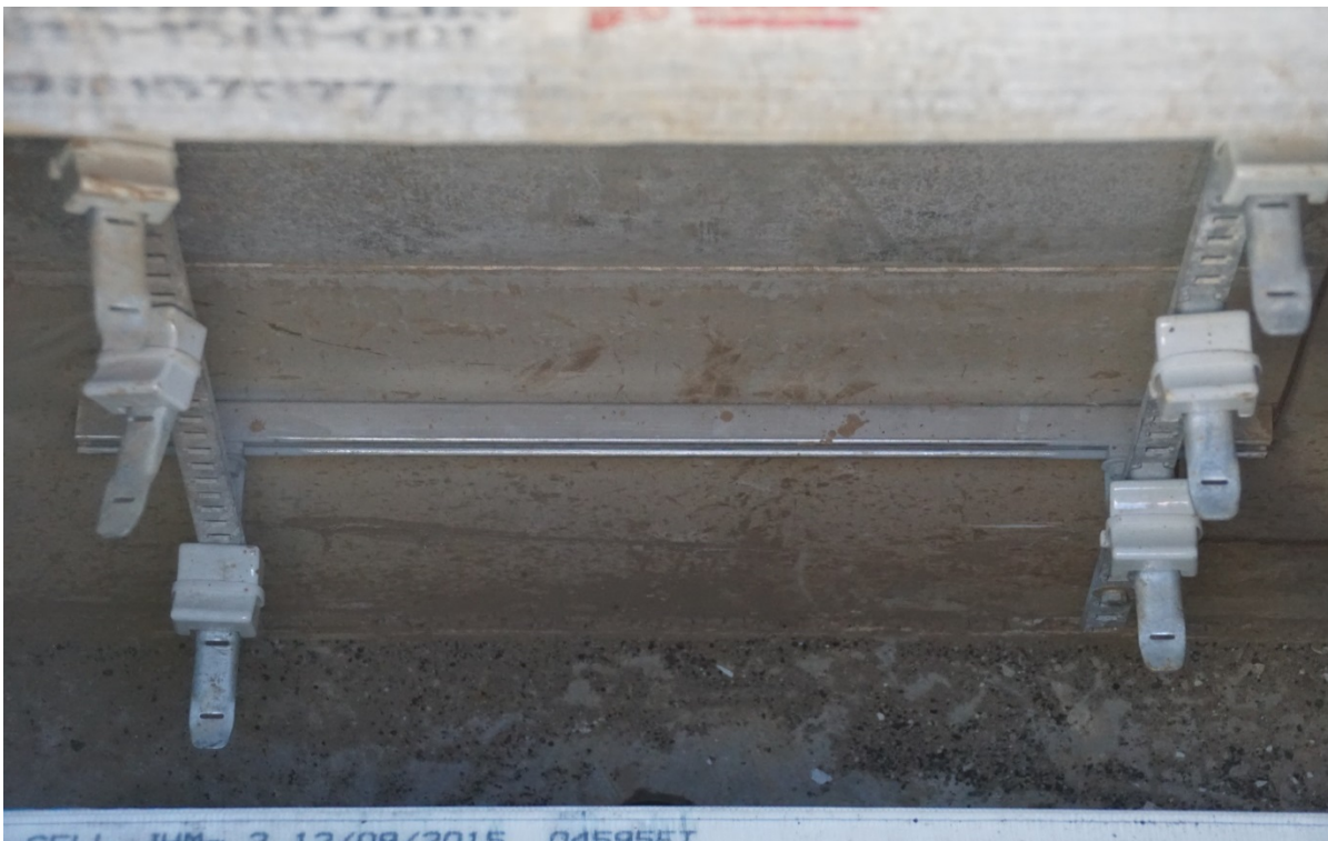
Maintenance Holes require cable mounting racks on both sides able to support 400 lbs each.
