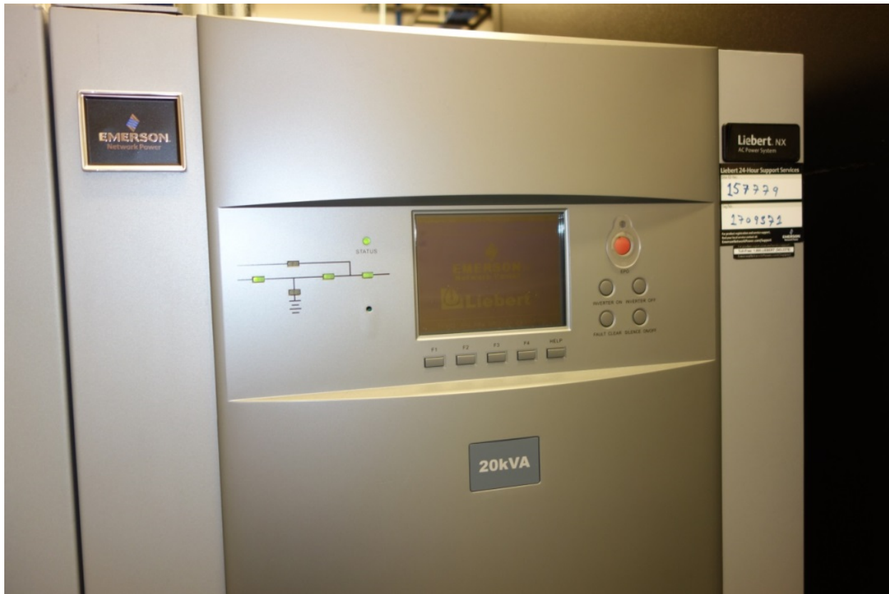
Close-up of a 20kVA Liebert UPS for a standard 6-cabinet IT Room.
