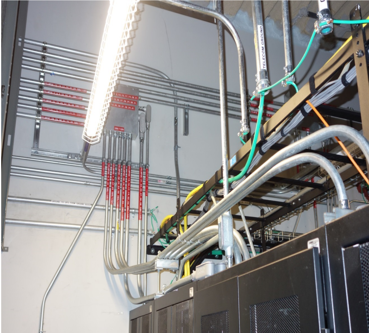
Electrical conduits feeding individual cabinets toward cabinet rear.
