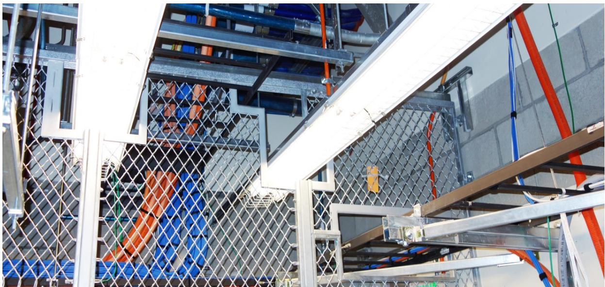
Divider wall enclosing light fixtures and ladder rack.
