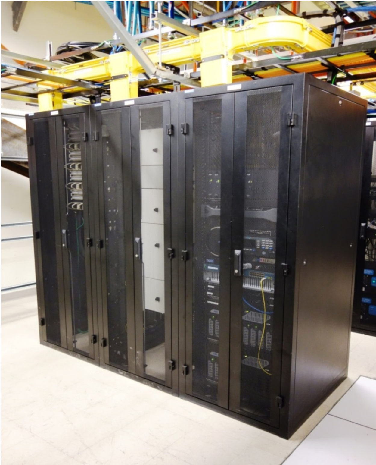
Existing IT Room shown with 2 rows of Damac cabinets.
