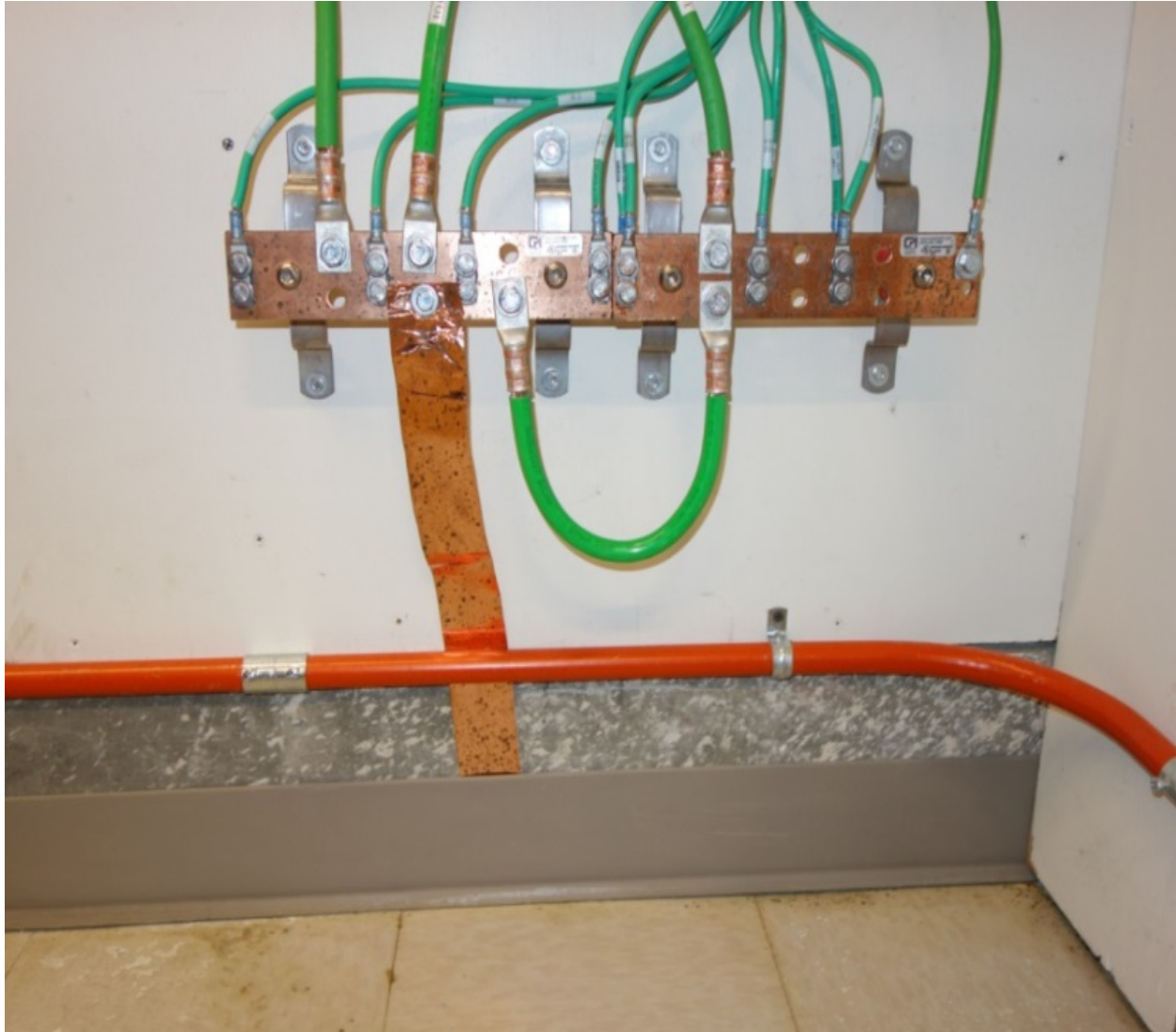
Copper bonding strap shown from floor tile to grounding bus bar.
