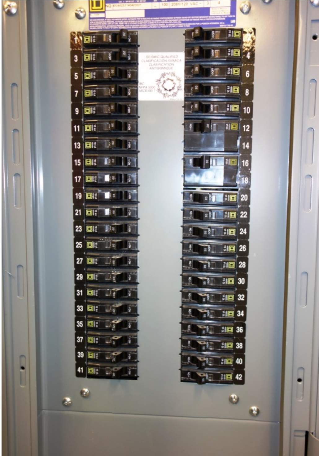
Fully populated breaker panels are required.
