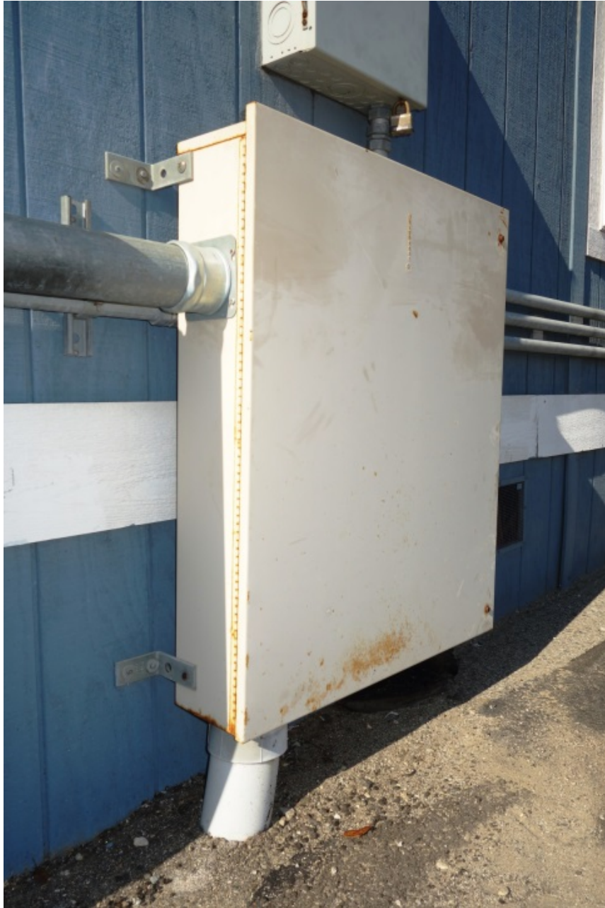
Legacy TE showing two 4-inch conduits on the left plus additional conduits on the right.
