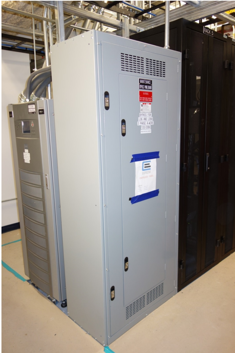
Maintenance Bypass for UPS shown.
