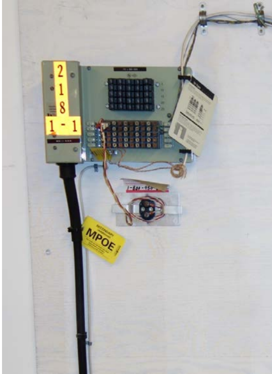
Small Copper Entrance Facility.
