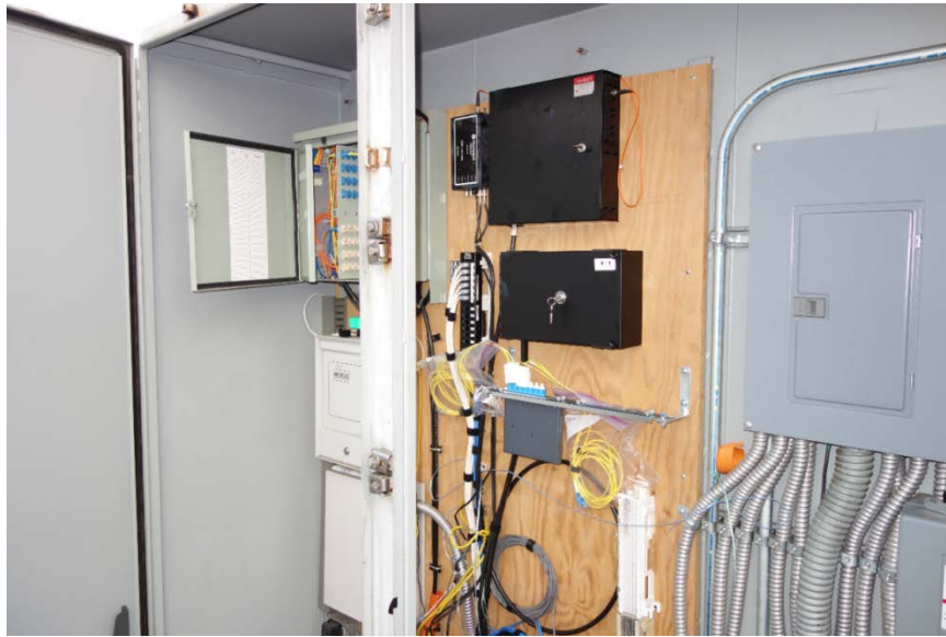
A legacy outdoor TE with plywood backboard - prior to the stainless steel requirements.
