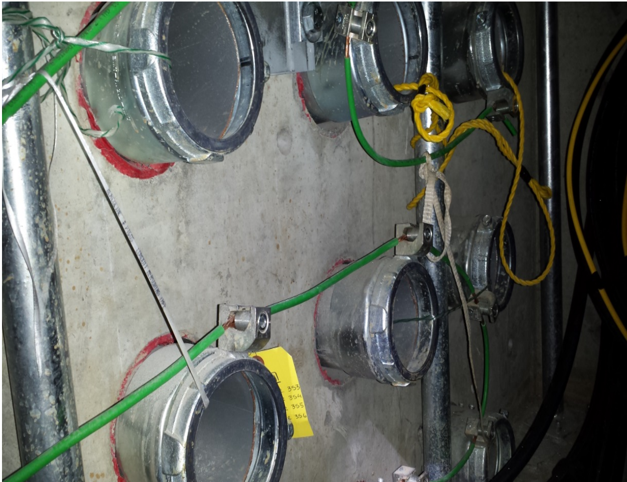
Empty conduits are shown with pull strings and ropes.
