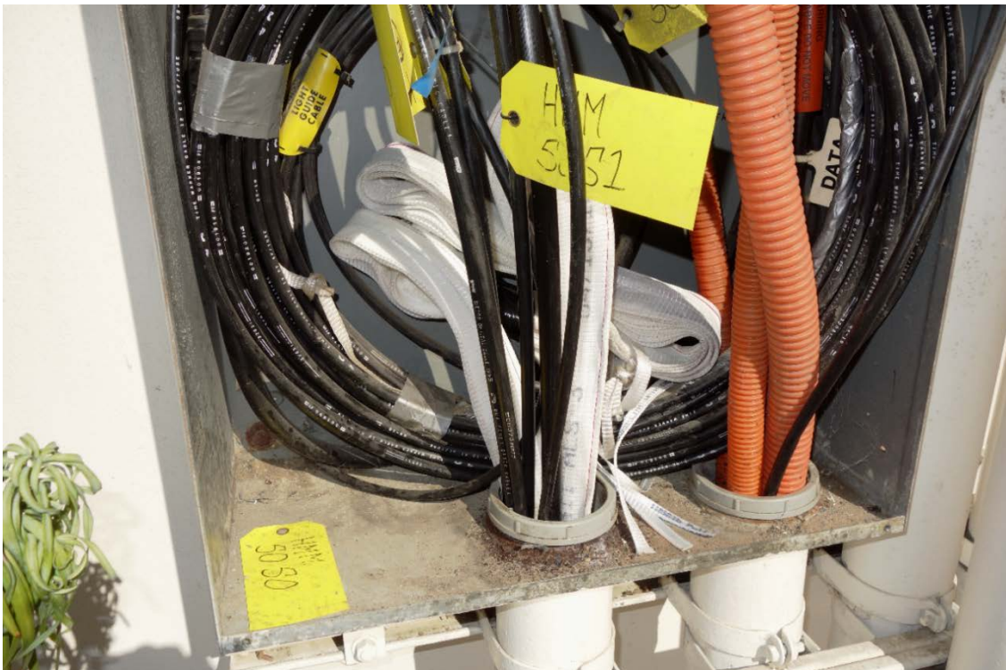
MaxSpace Recovery process: Three innerducts have been removed and two Maxcell's installed.
