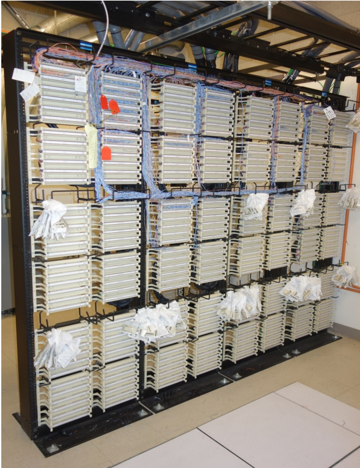
Front View of an MPOE MDF shown with racks of 110 Blocks for Copper BD.
