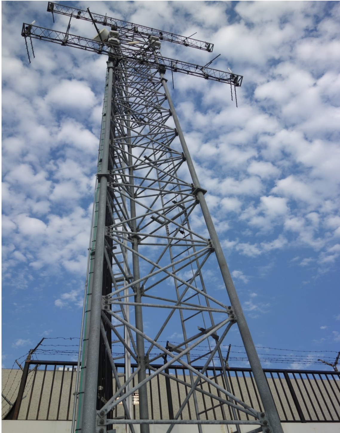
Triangular antenna tower with ladder and safety fall arrest.
