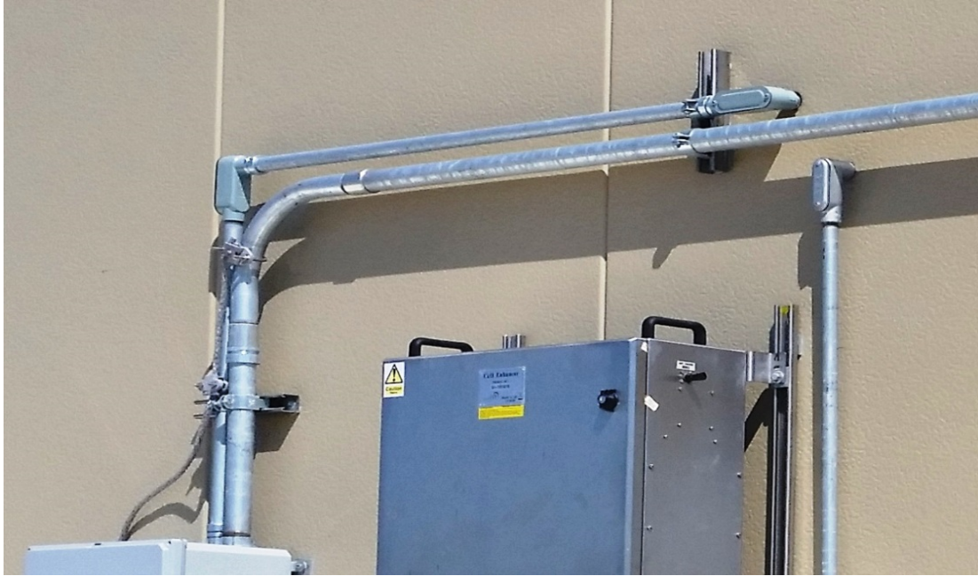
Conduit bodies/condulets used for copper cables.
