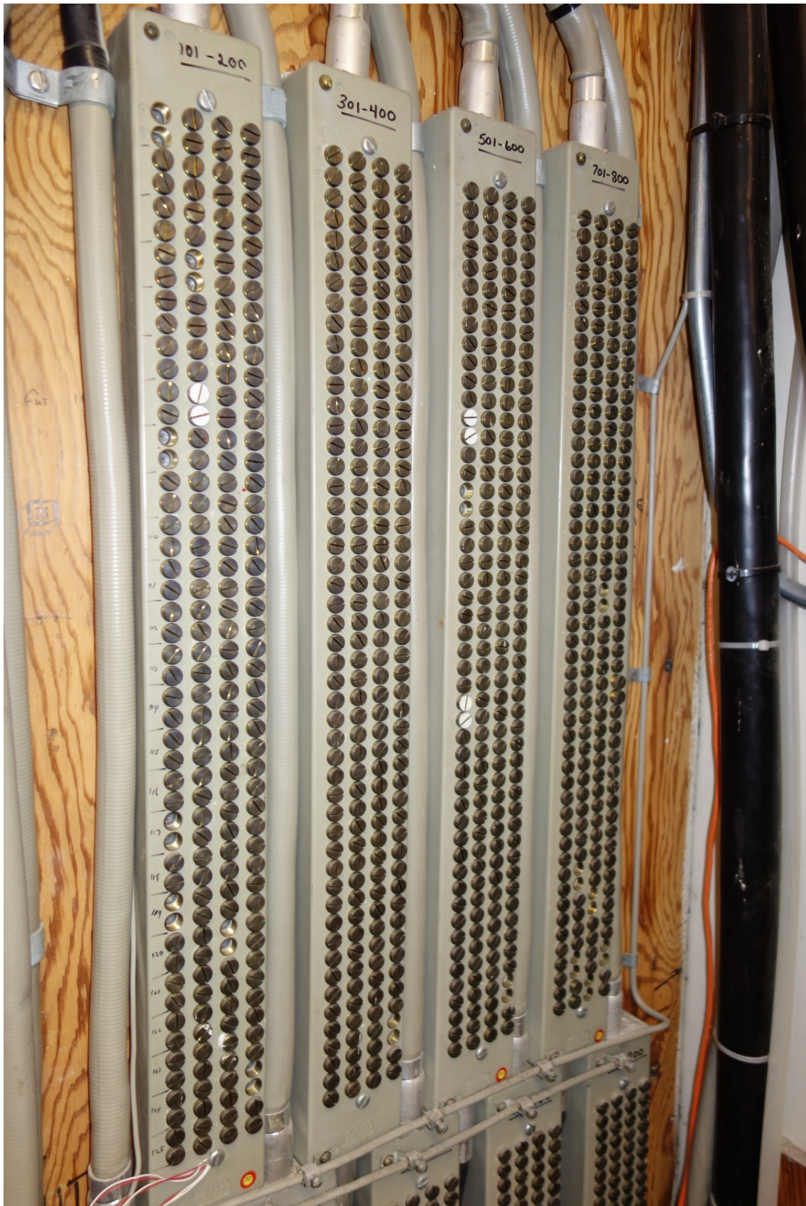
Protector blocks for a 1600-pair Cat 3 copper cable.
