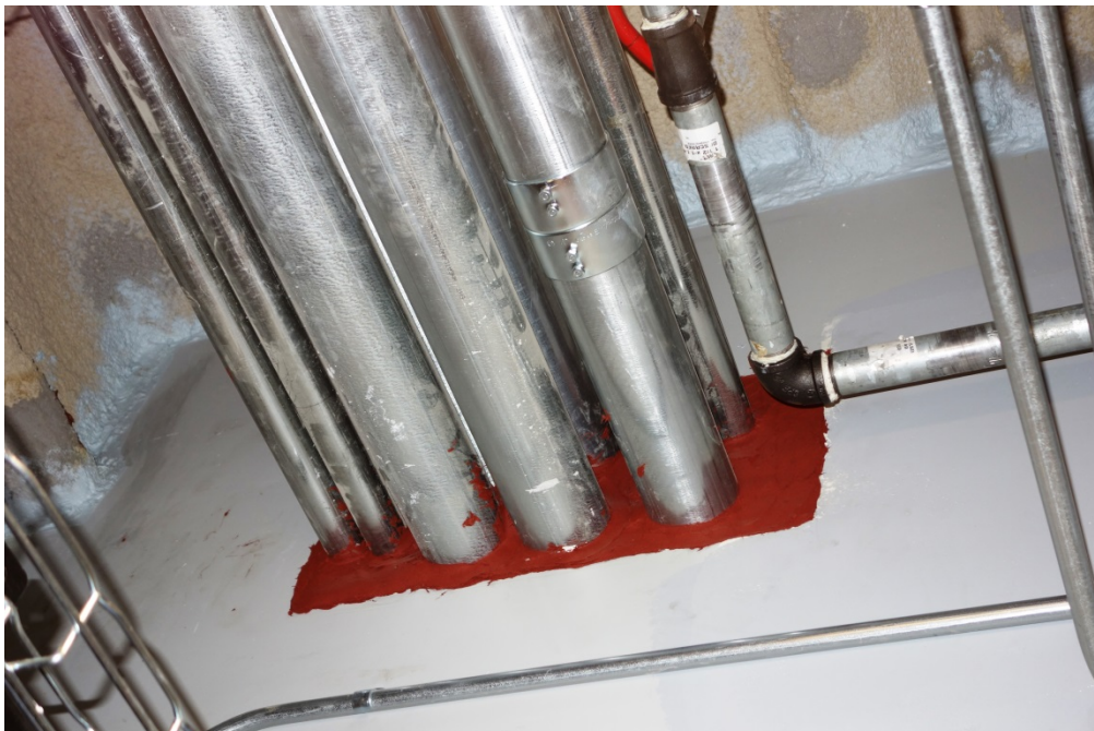
Firestop putty around all individual conduits in a common wall entry.
