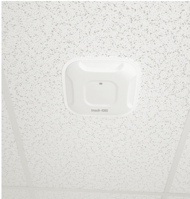
A/P mounted within ceiling tile on the suspended ceiling T-Bar.
