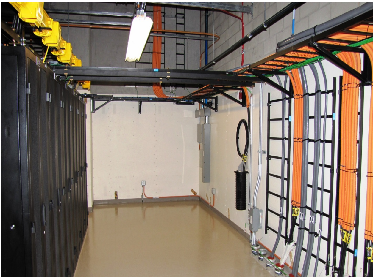
In IT Rooms, vertical Ladder Rack is required to secure cables that transition to floor conduits.
