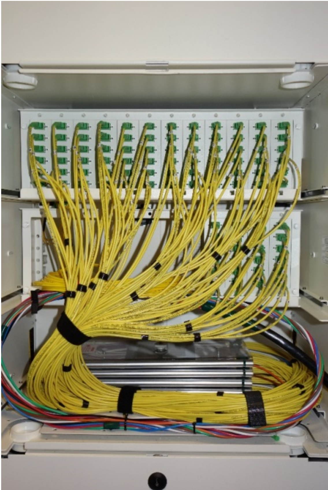
Pigtails of the same color shall be labeled with the strand number.
