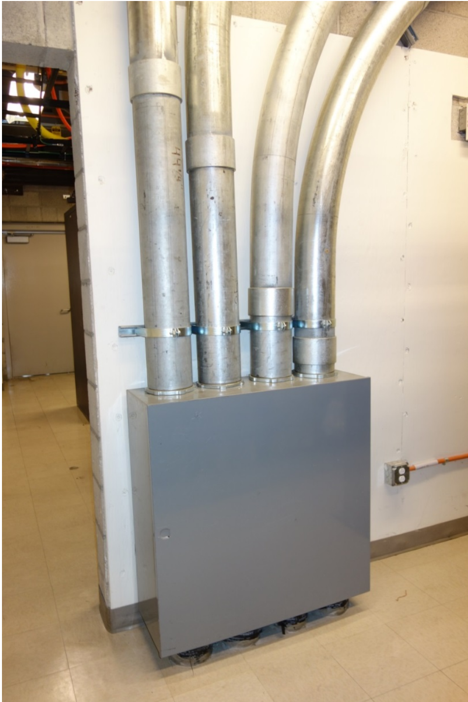
An Entrance facility pull box.
