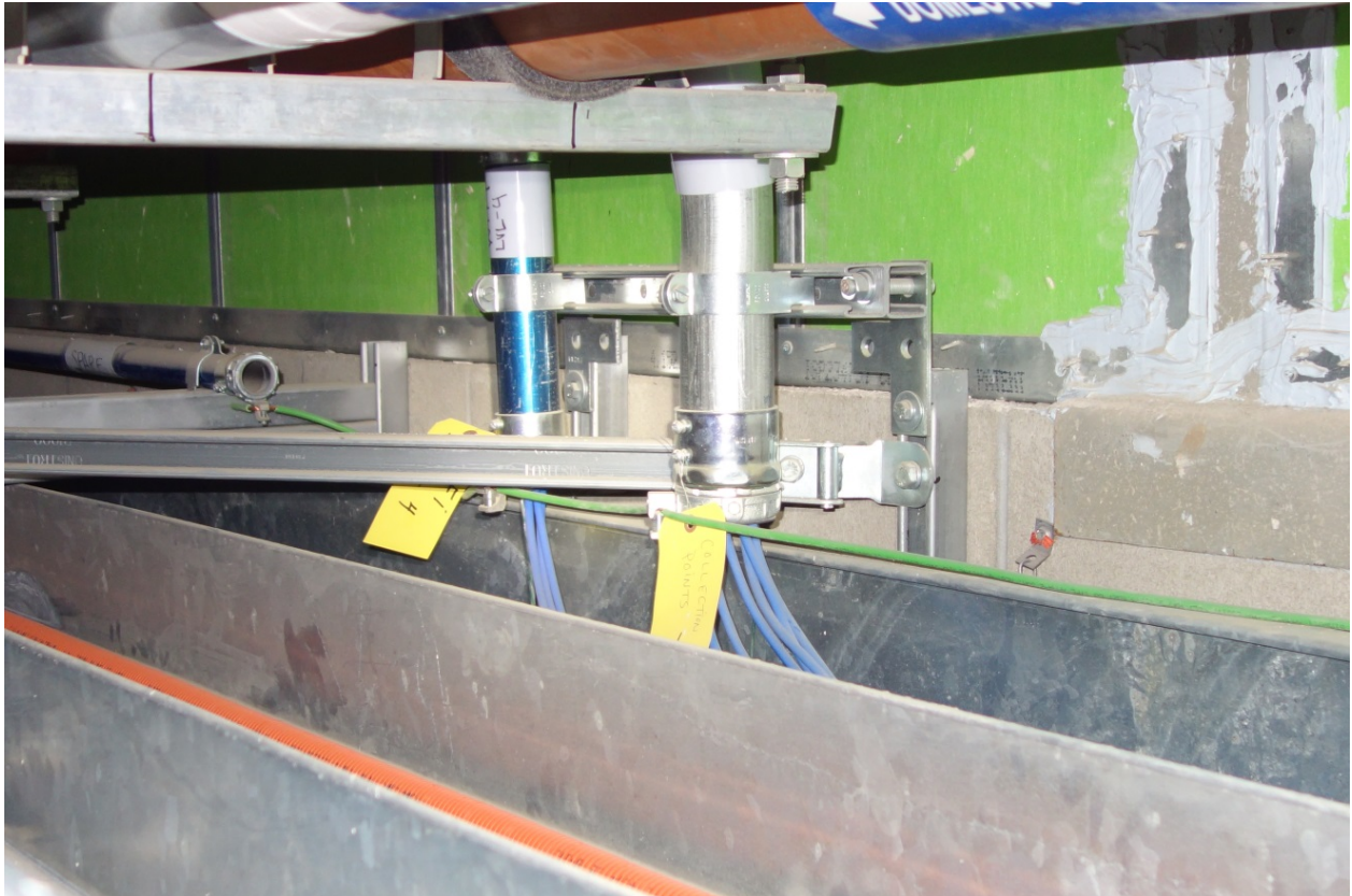
Last mile conduit into cabletray from tenant leasehold shown.
