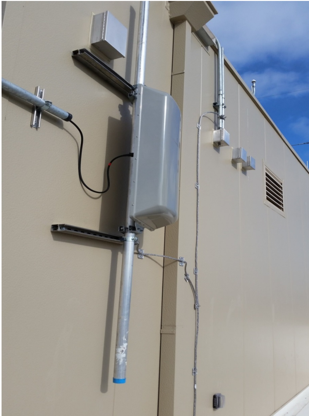
Wall-mounted antenna higher than 6-feet.
