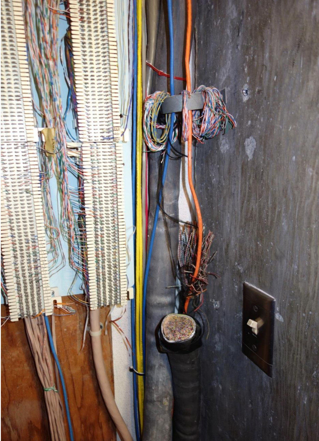
Cut cables shall not be abandoned in place.
