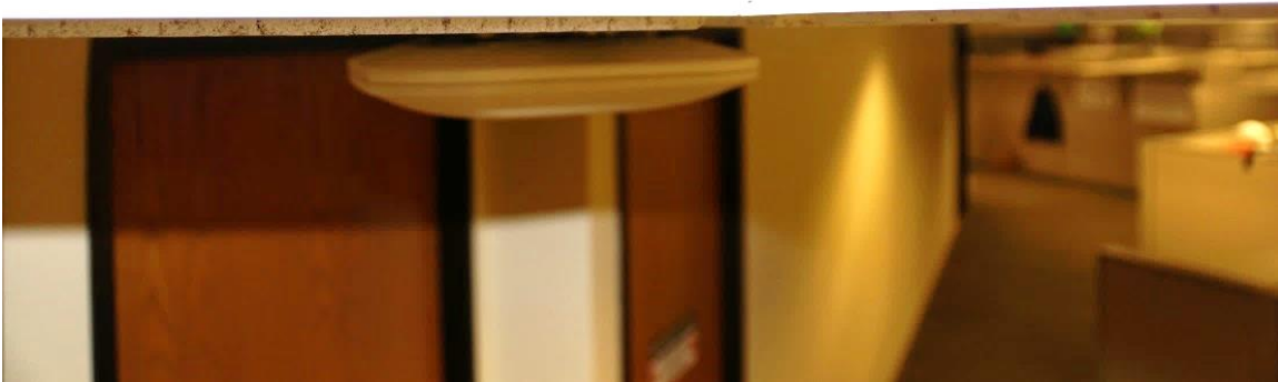
A/P cable fed from above-ceiling through a hole in the ceiling tile.
