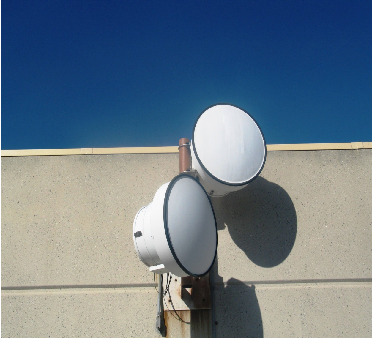
Wall-mounted antenna are shown.
