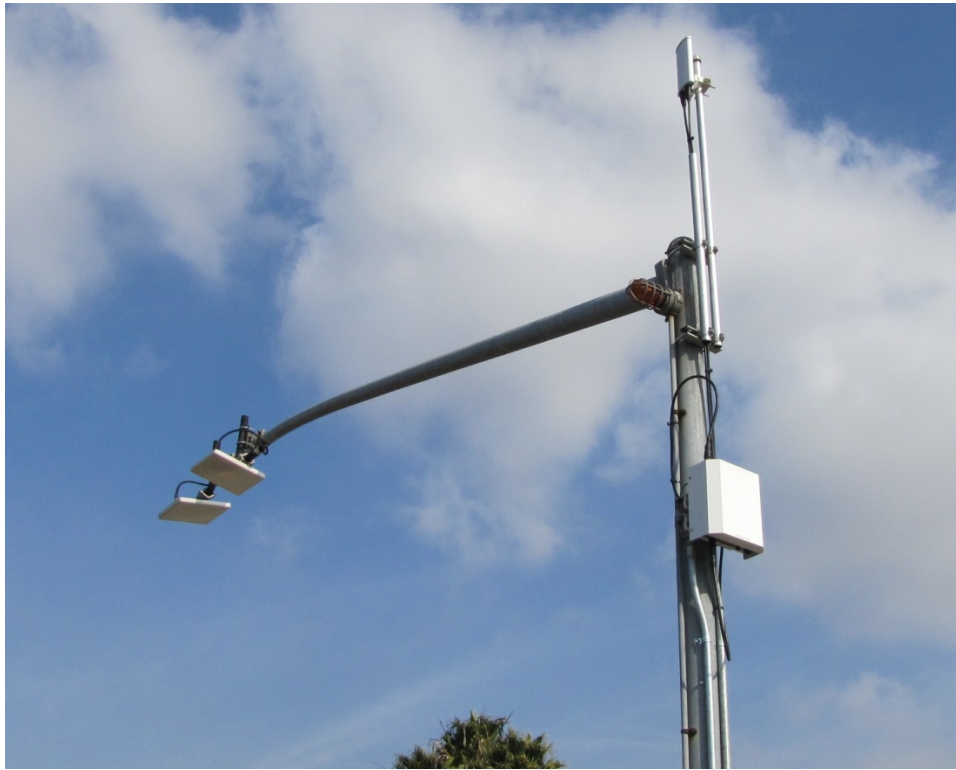
Cable protected up antenna pole.
