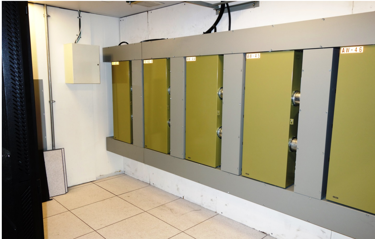
A bank of wall-mounted fiber patch panels shown with interconnecting wireway.
