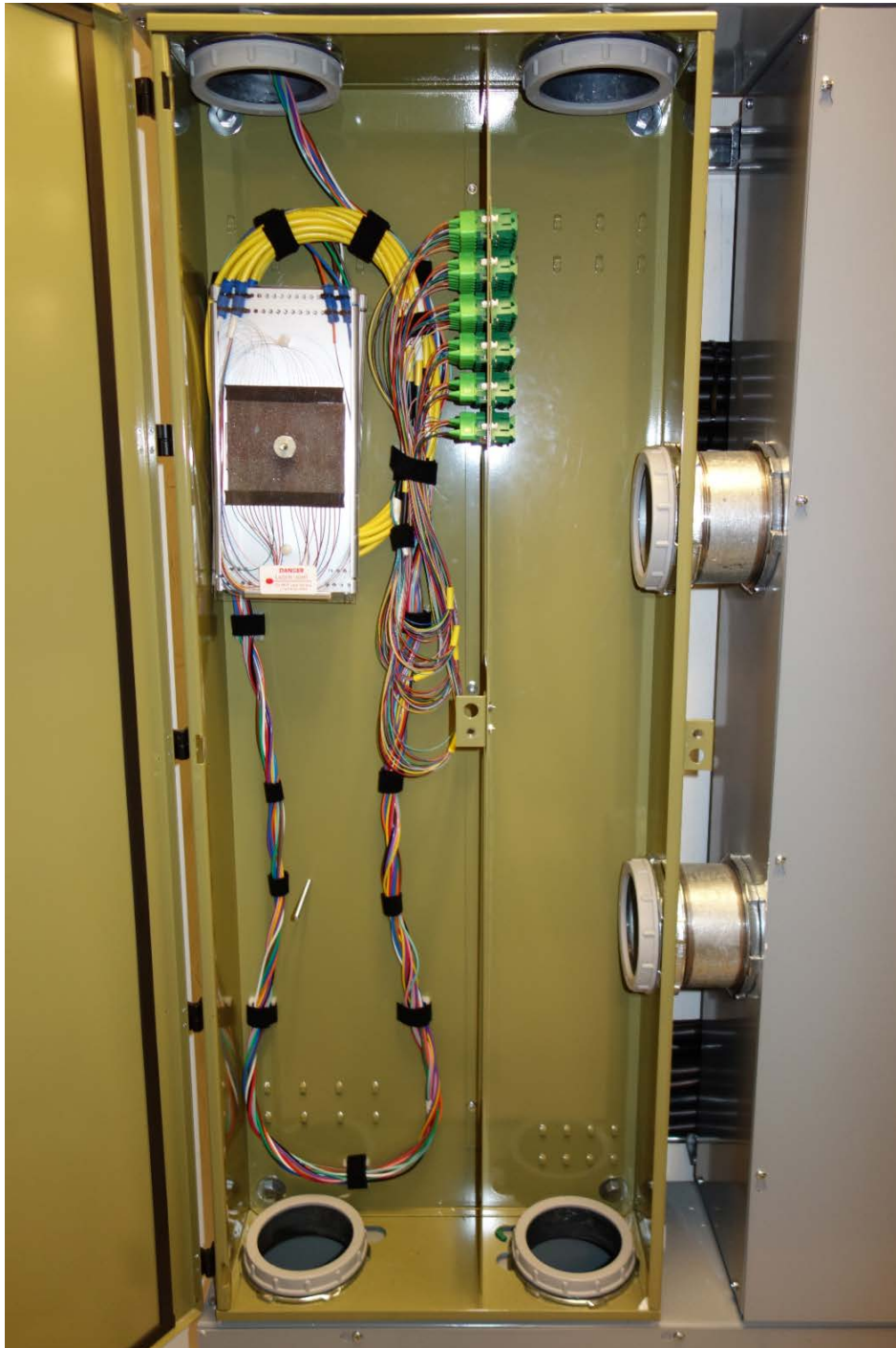
Wall-mount FPP's shall have wireway and six 4-inch chase nipples installed as shown.
