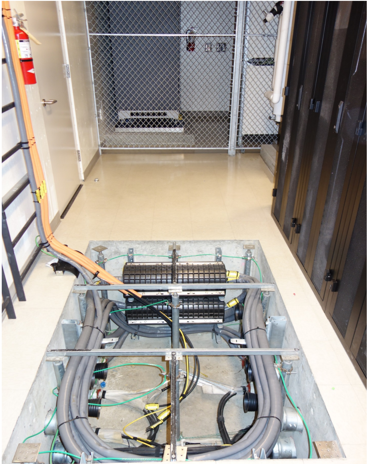
Conduit wells shall be nest to the IT Room wall so that cables are not a trip hazard as shown here.
