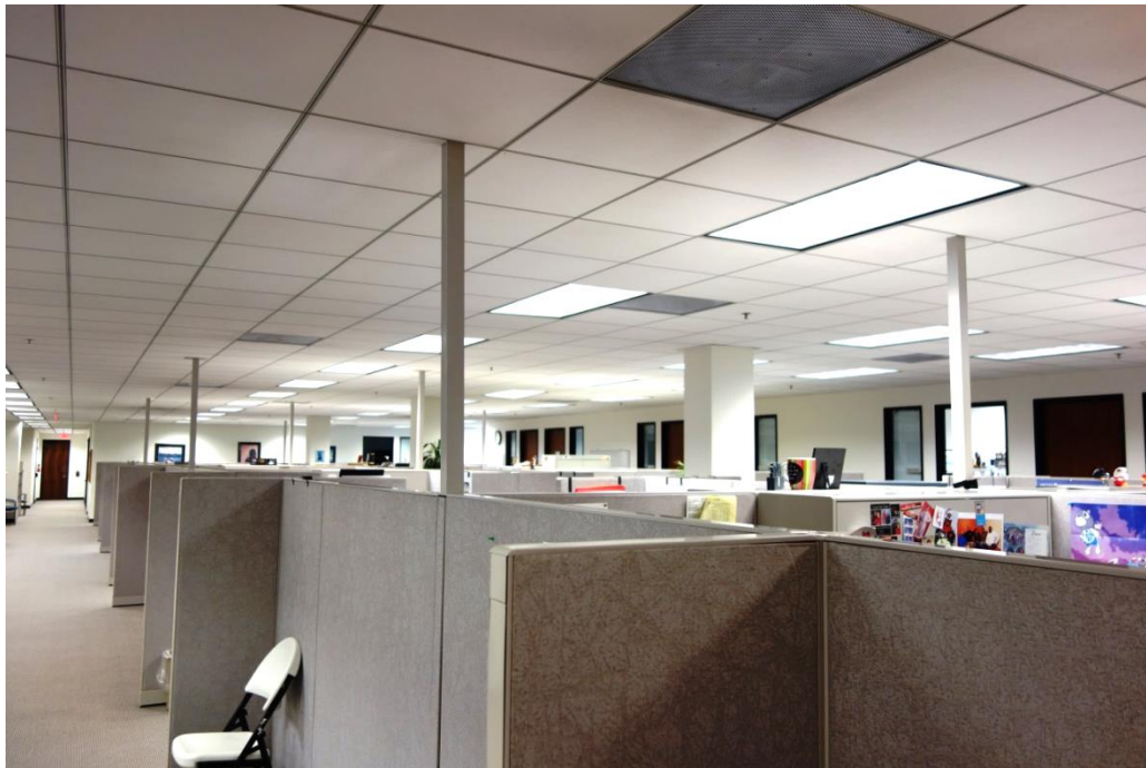
Cubicle islands may be fed from split power/comm. poles.
