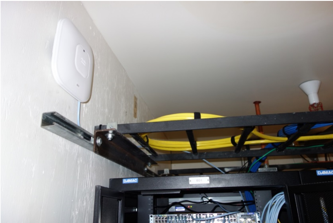
AP mounted in an IT Room on the side-wall.
