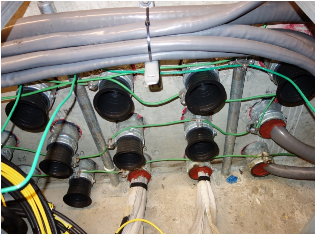
Conduit well showing cable support, fabric innerduct, firestop, and conduit plugs.
