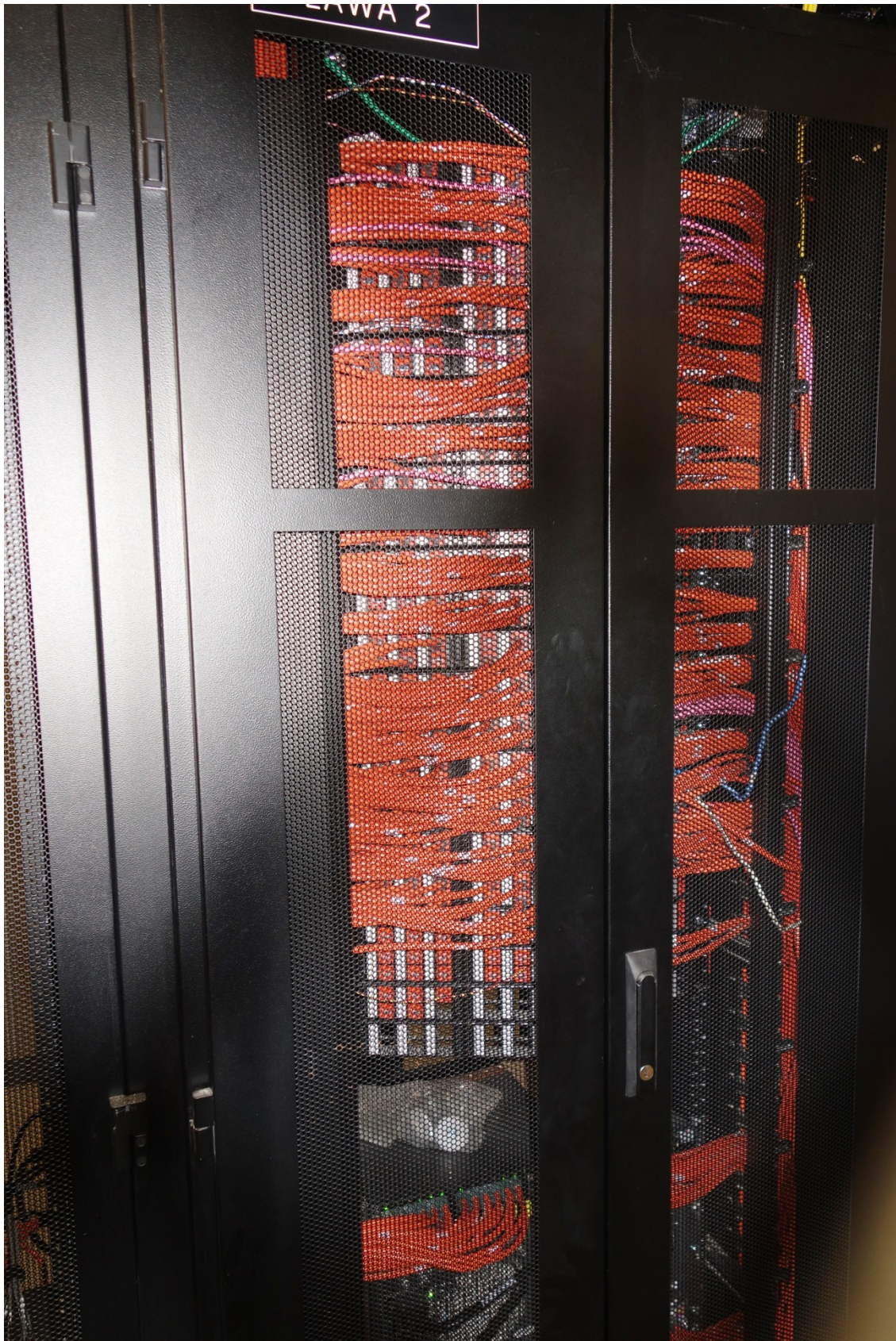
A through-cabinet view of CAT 6A cables terminated per LAWA standards.
