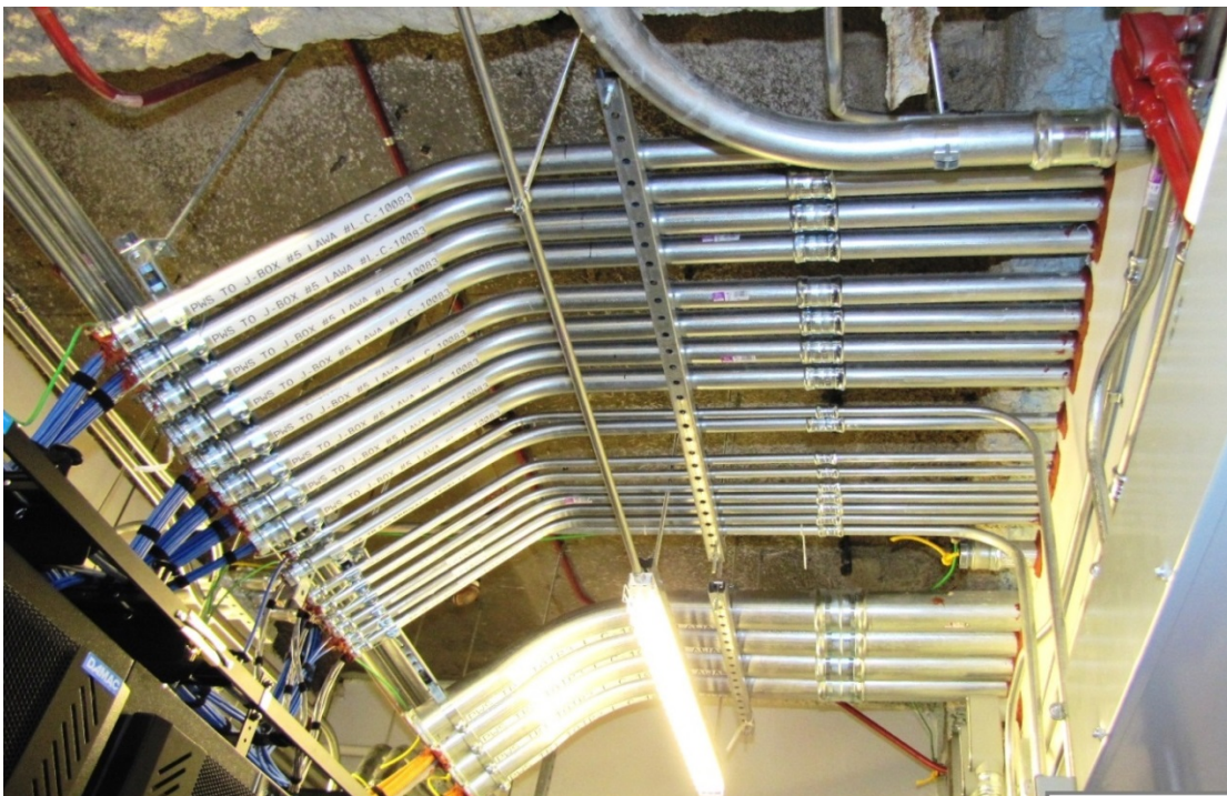
A neat professionally-installed and labeled horizontal conduit bank with bushings is shown.
