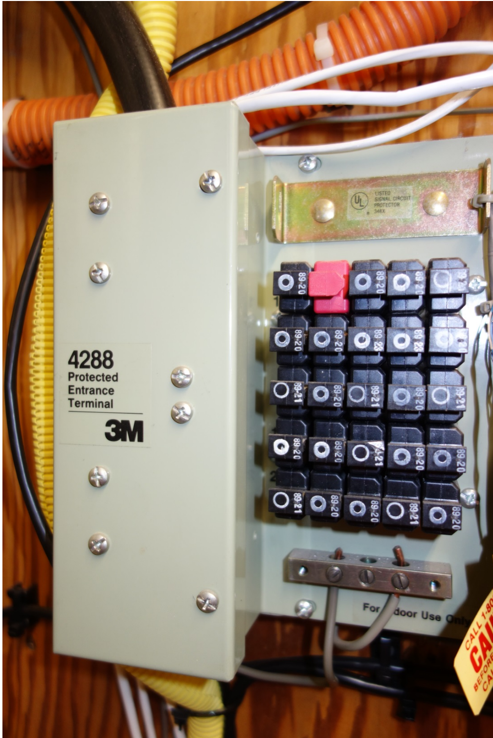
Protector blocks for a 25-pair Cat 3 copper cable.
