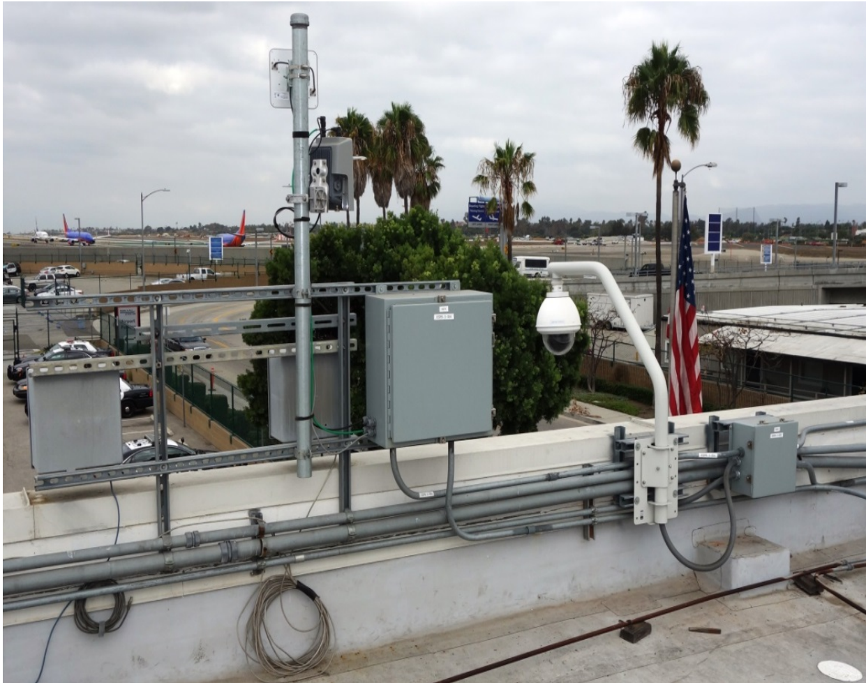
Parapet wall antenna and conduit pathway.
