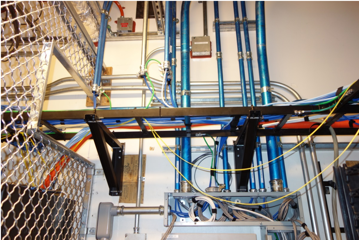
Wireway is shown with cable slack loops for an IT system.
