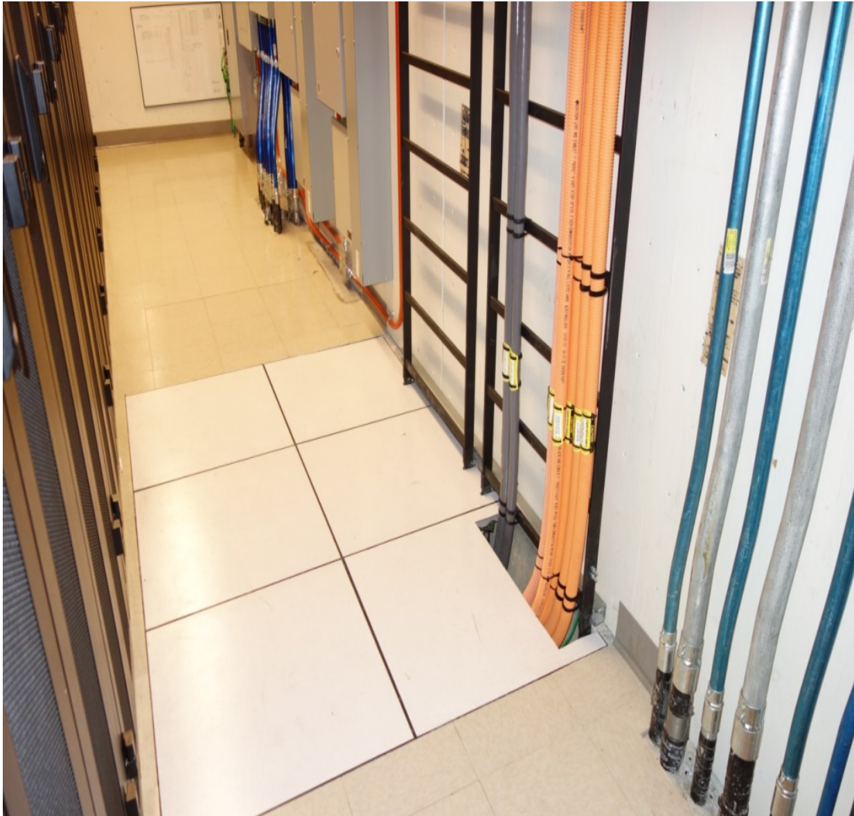
A conduit well shown adjacent to the IT Room wall with access through a cutout tile.
