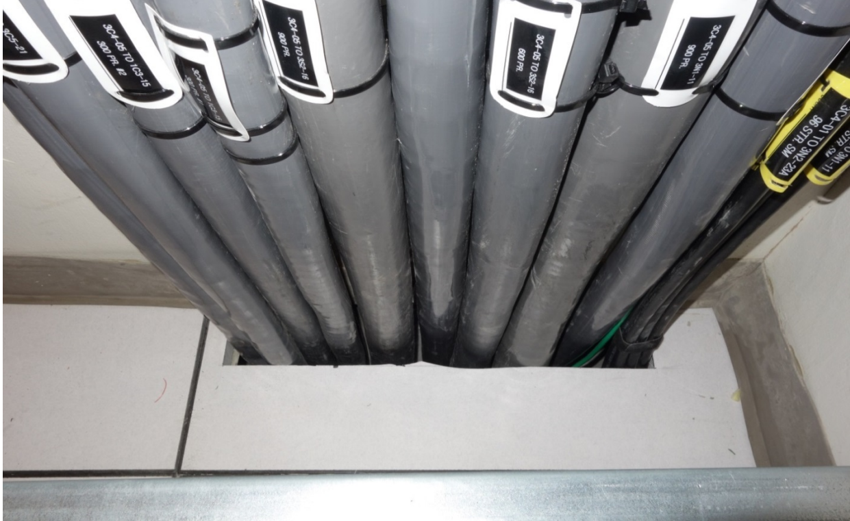
Backbone inside plant CAT 3 copper cables being distributed from an MPOE to local IT Rooms.
