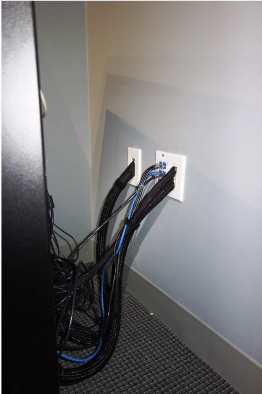
WAO's shown with jumpers and split-loom-covered cables.
