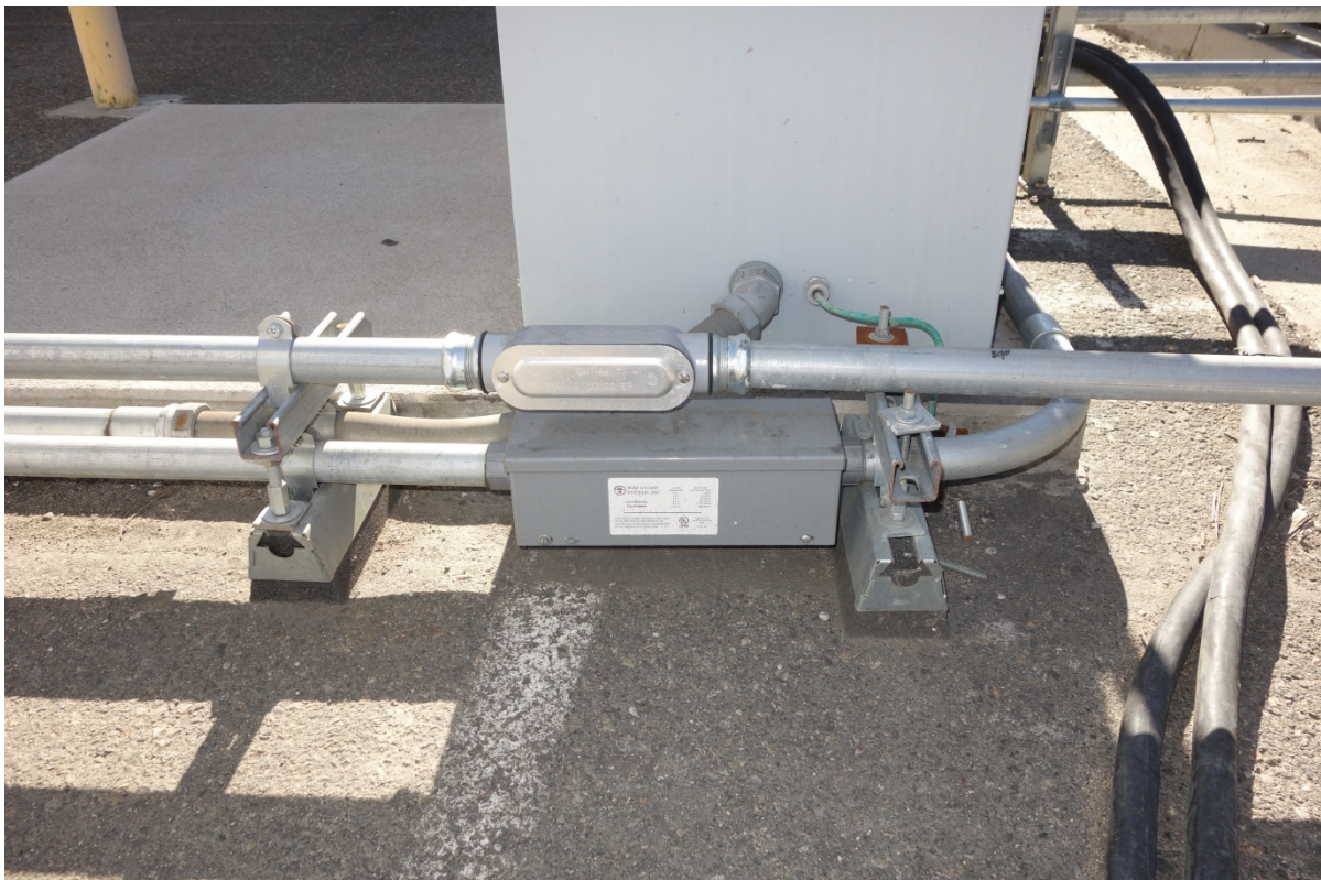
A temporary transformer using galvanized rigid conduit is shown.
