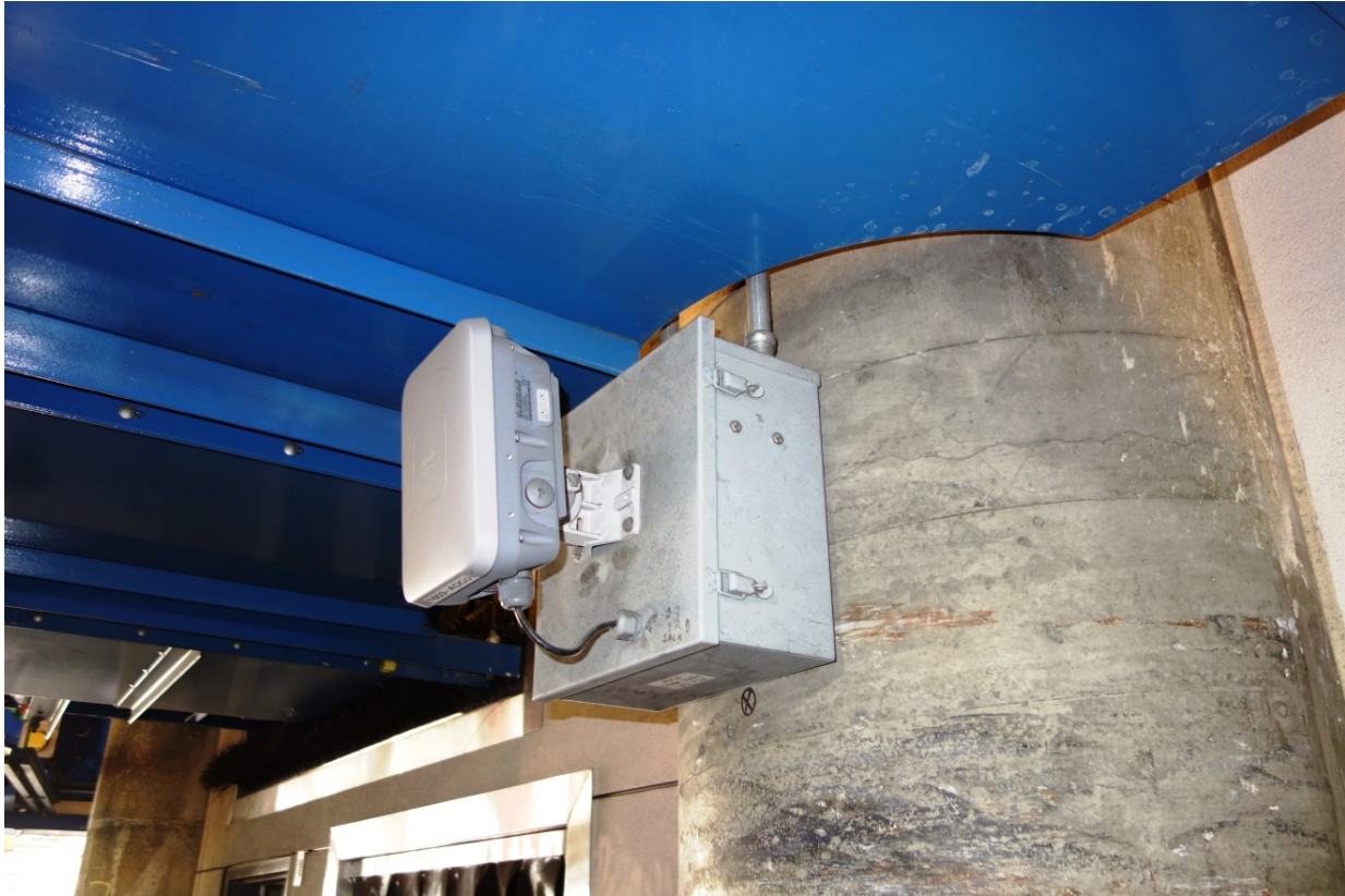
An outdoor A/P is shown mounted on a support column.
