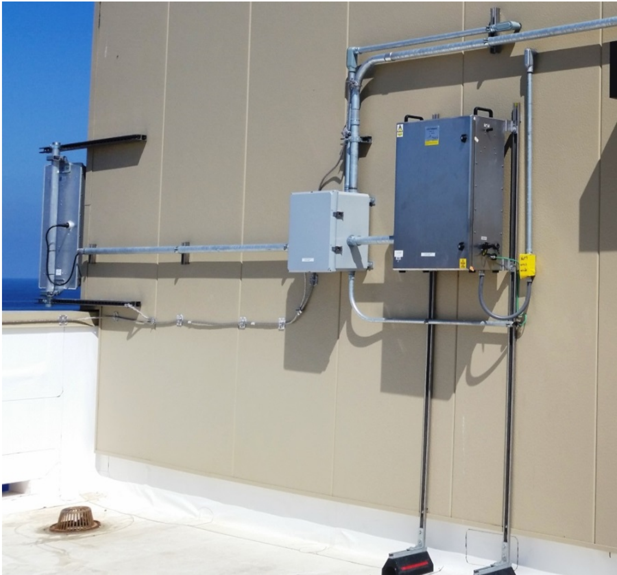
Wall-mount antenna and conduit pathway.
