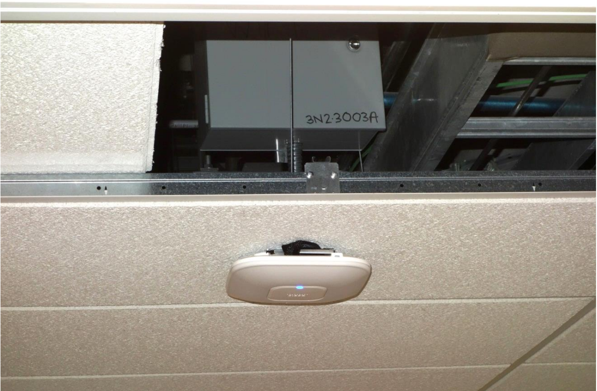
A legacy A/P mounted in the center of a suspended ceiling tile prior to T-Bar mounting required.
