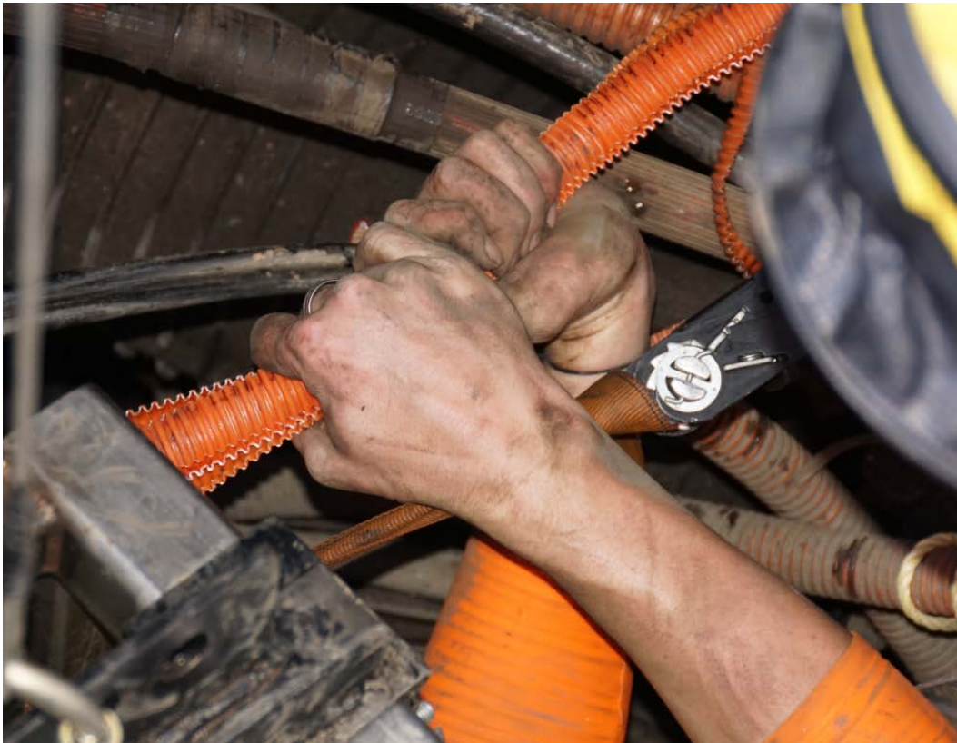
MaxSpace Recovery process: The first innerduct is being split and pulled out of the ductbank.
