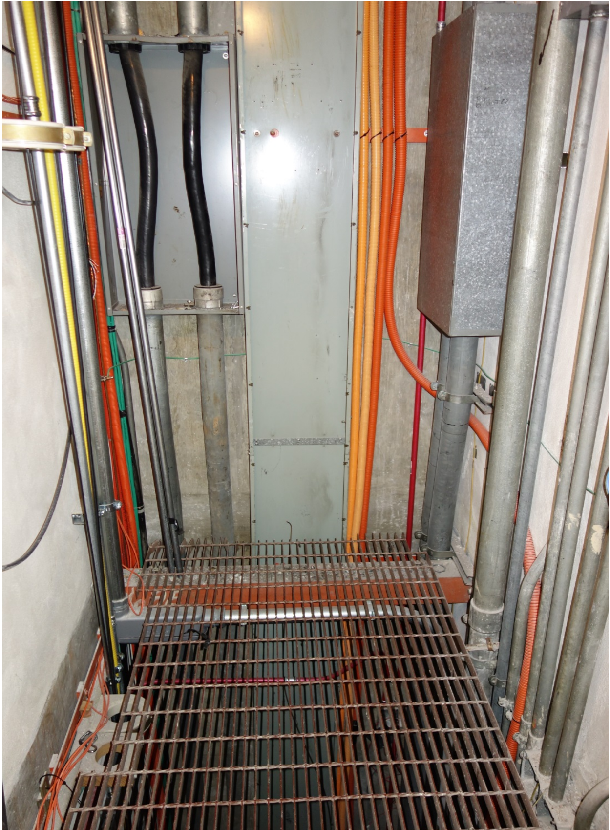
A conduit chase (riser room) as a dedicated pathway in a large facility is shown.
