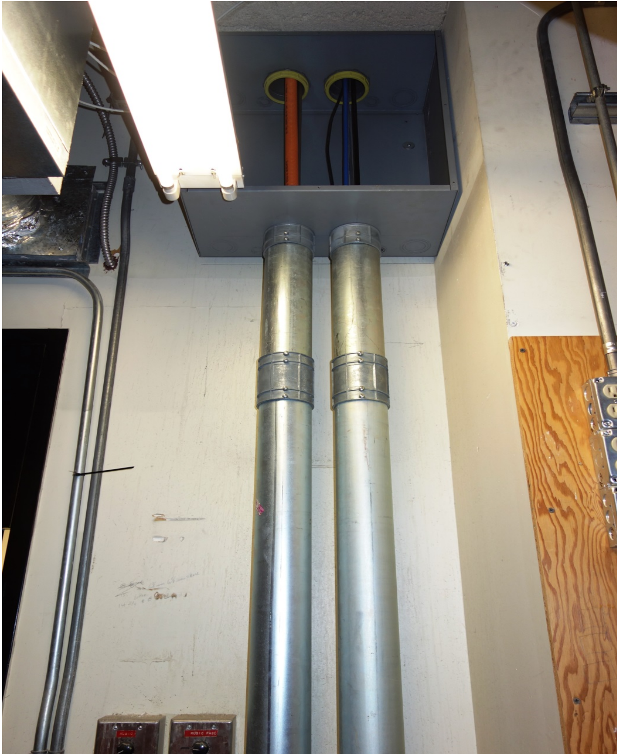
A small conduit riser shown with large pull box.
