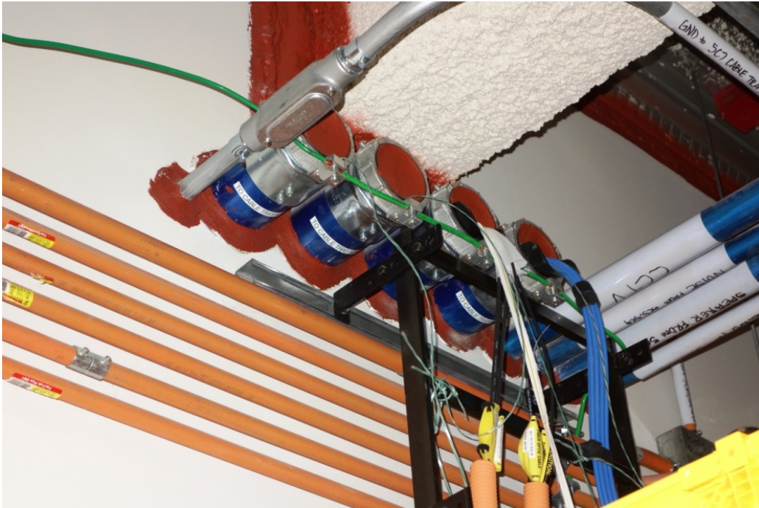
Firestop putty is shown around all Horizontal Distribution conduits.
