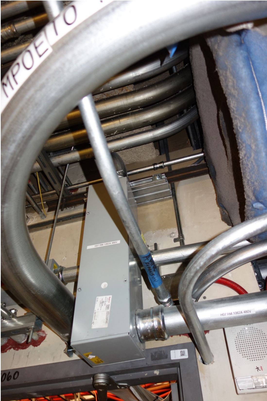
Pull box for a 90-degree conduit direction change.
