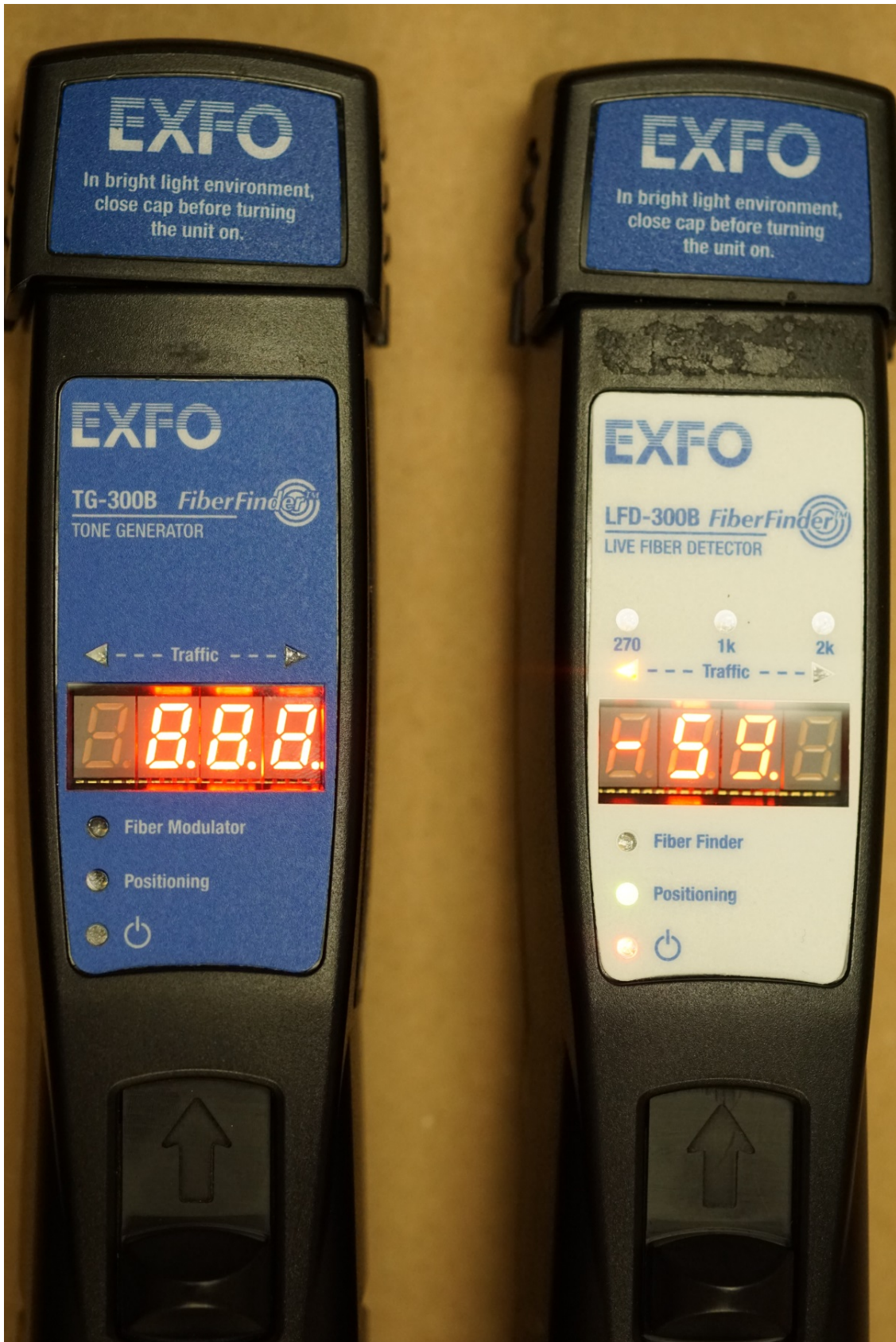
A live fiber circuit finder is required when verifying the correct circuit to work on.
