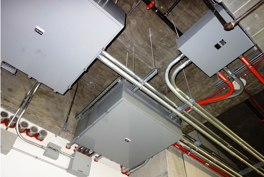
Indoor pull boxes that are 24-inches square or greater shall have piano-hinge covers.
