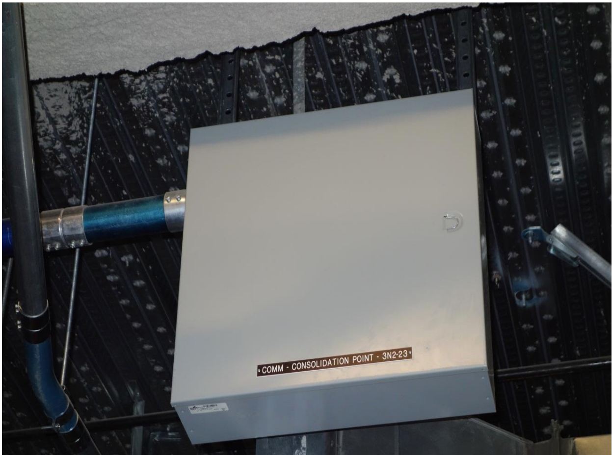
Consolidations Points may be installed in separate junction boxes in the ceiling.
