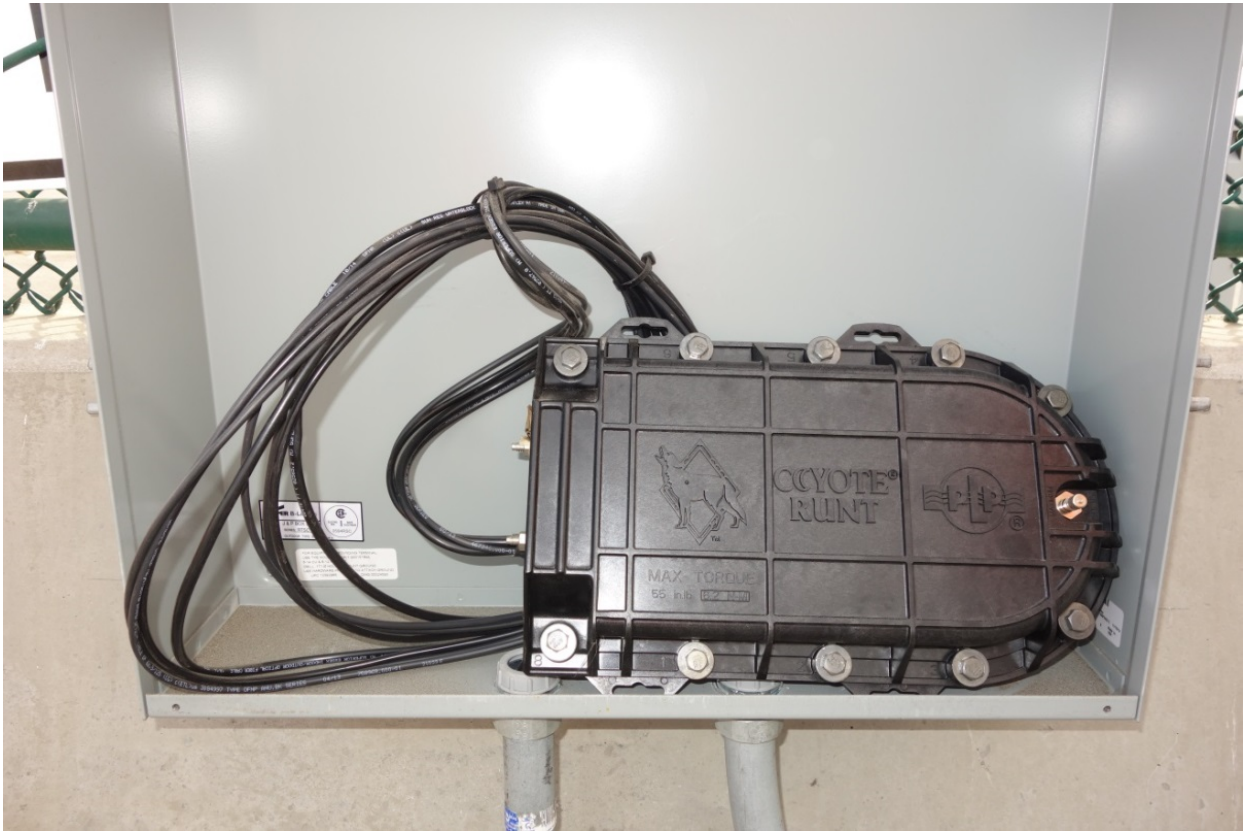
An intermediate outdoor splice case on a long fiber run shown in a junction box.
