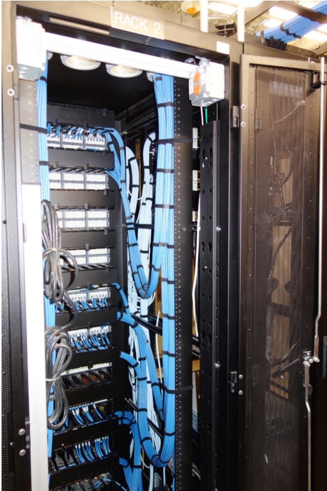
CAT 6A cable slack loops installed per LAWA standards.
