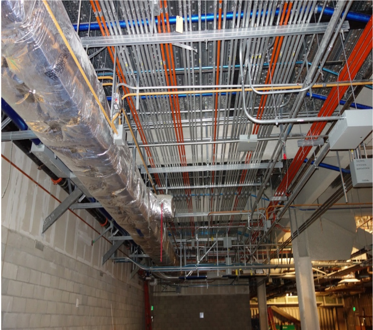
A neat and professional conduit installation.
