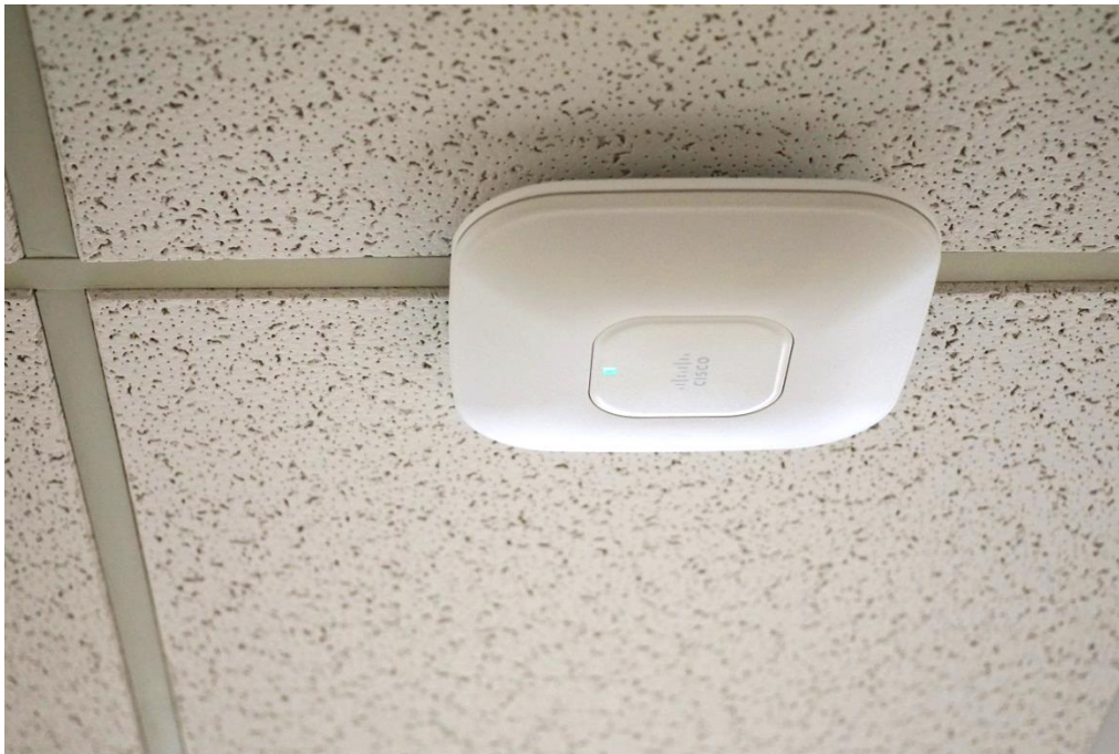
A/P mounted on suspended ceiling T-Bar.
