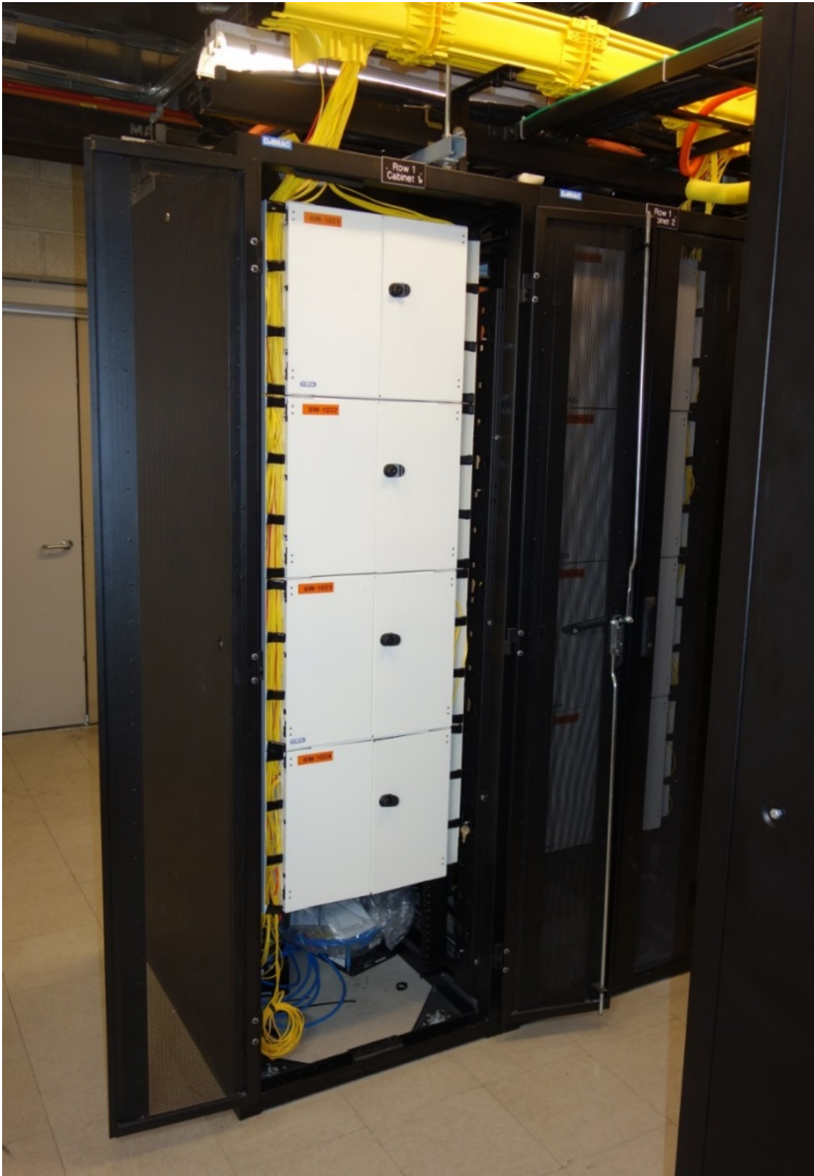
Fiber patch panels shall be mounted together within cabinets.
