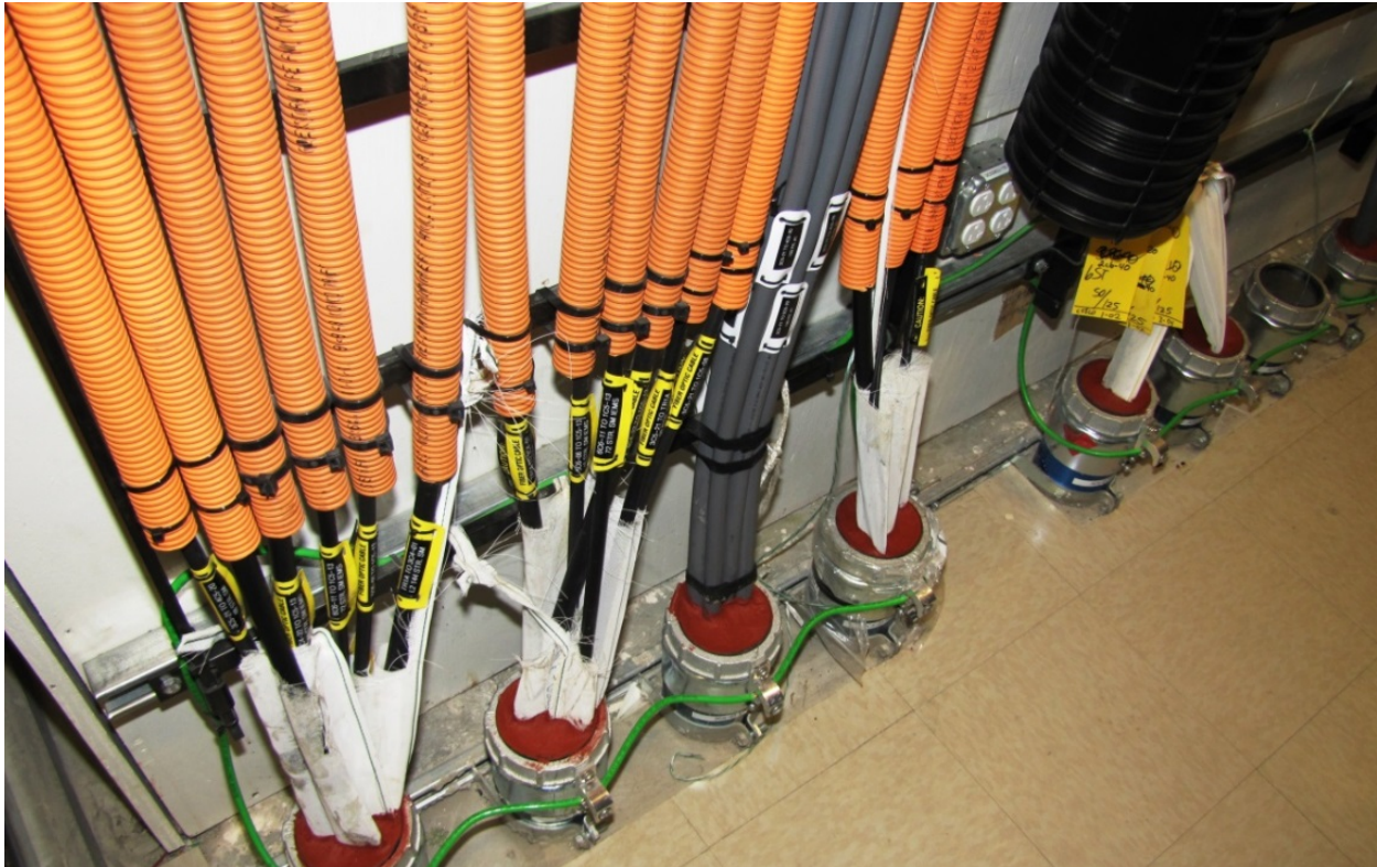
The transition from HDPE innerduct to Maxcell fabric innerduct within conduits is shown.
