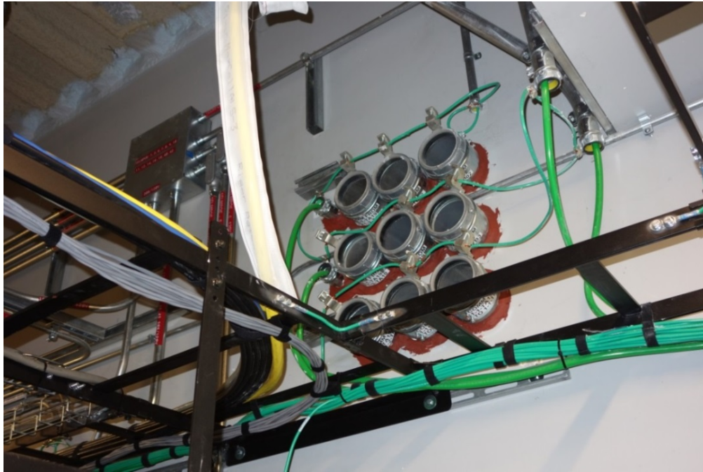
Firestop putty around all individual wall penetrations by conduit.
