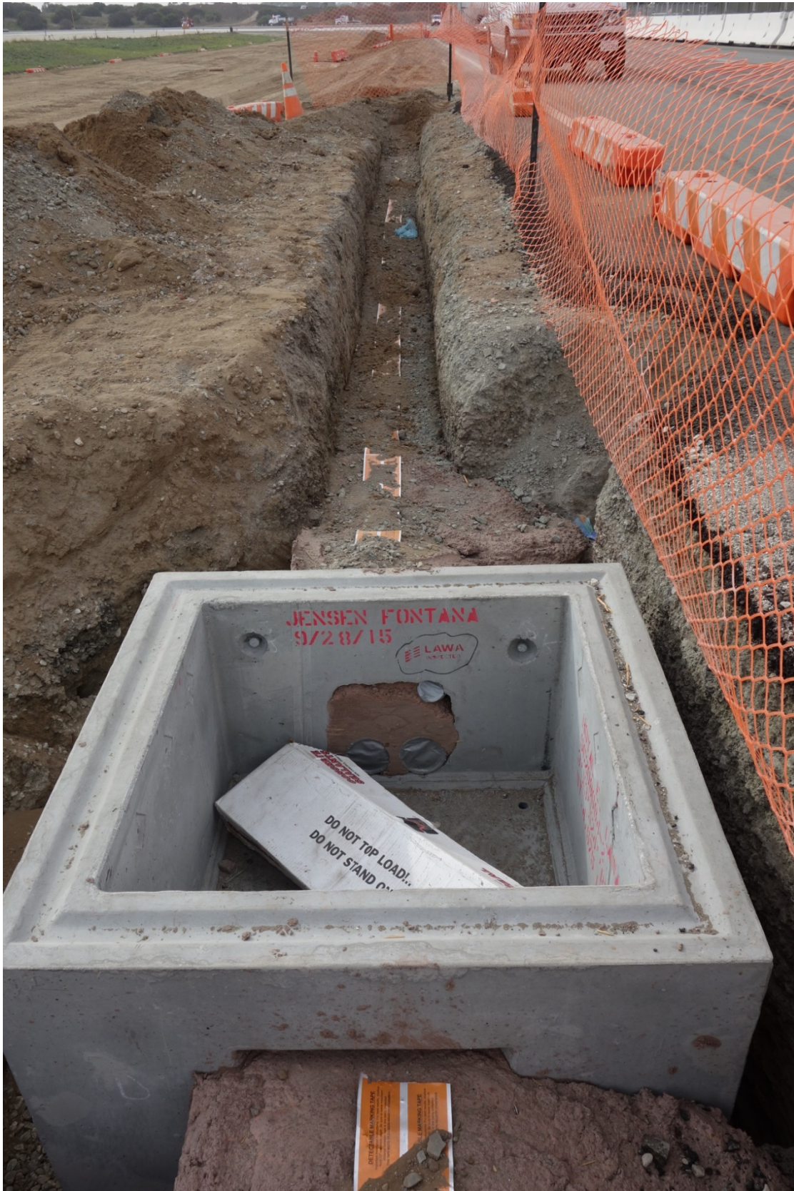
A ductbank using PVC concrete-encased conduits is shown with detectable I.D. tape.
