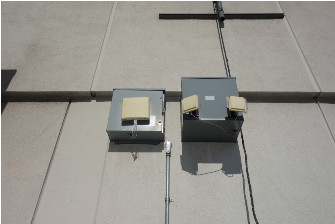
Multiple AP's are shown mounted on an exterior wall.
