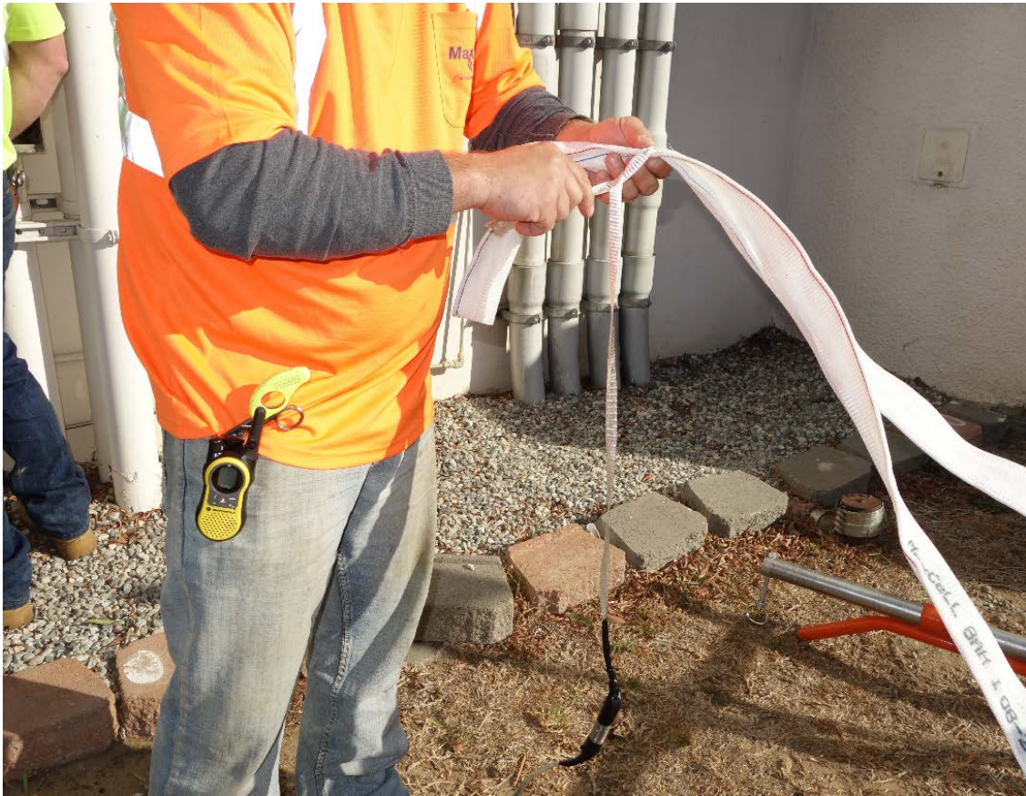
MaxSpace Recovery process: The fabric innerduct is being prepared to replace the HDPE.
