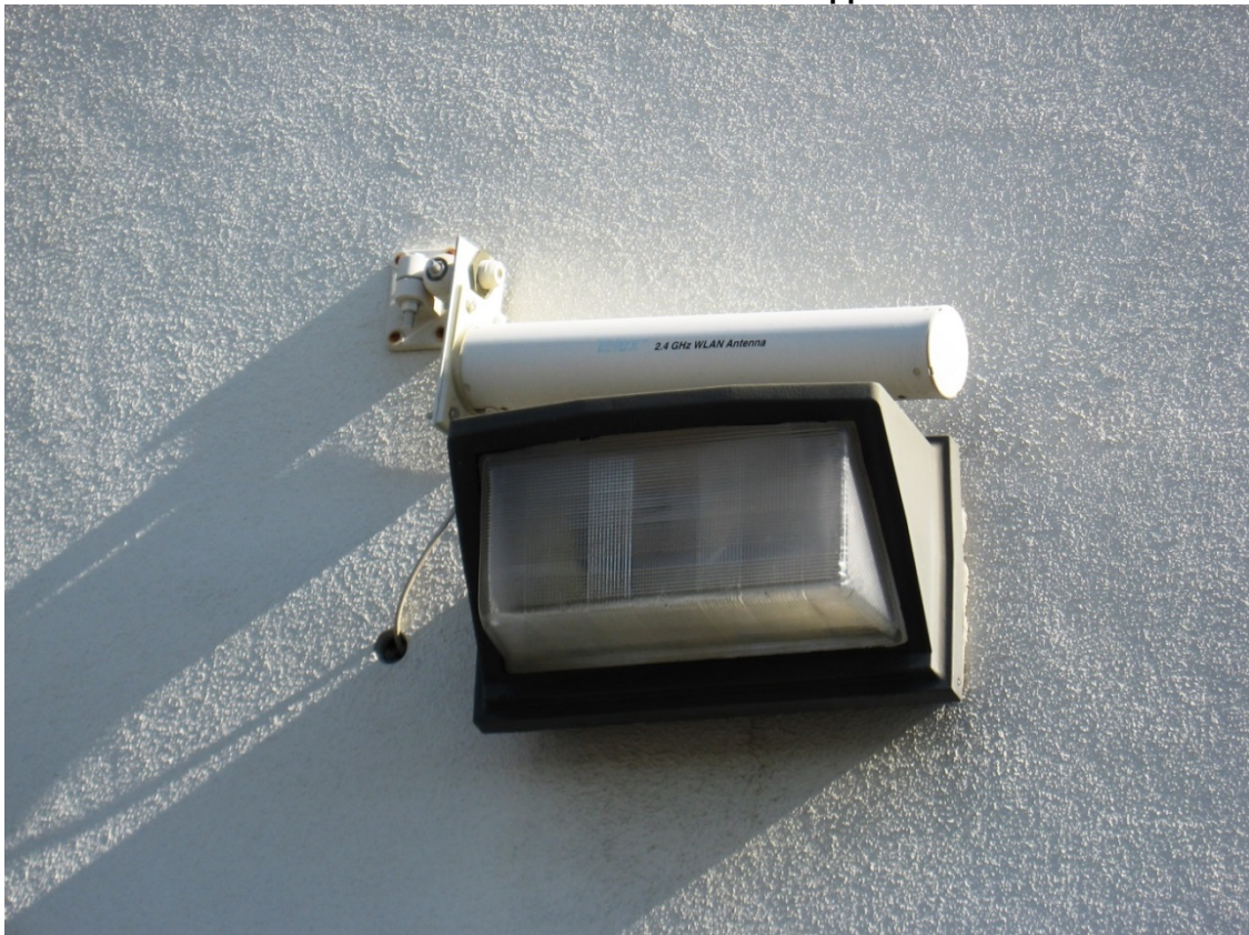
A single A/P is shown mounted on an exterior wall.
