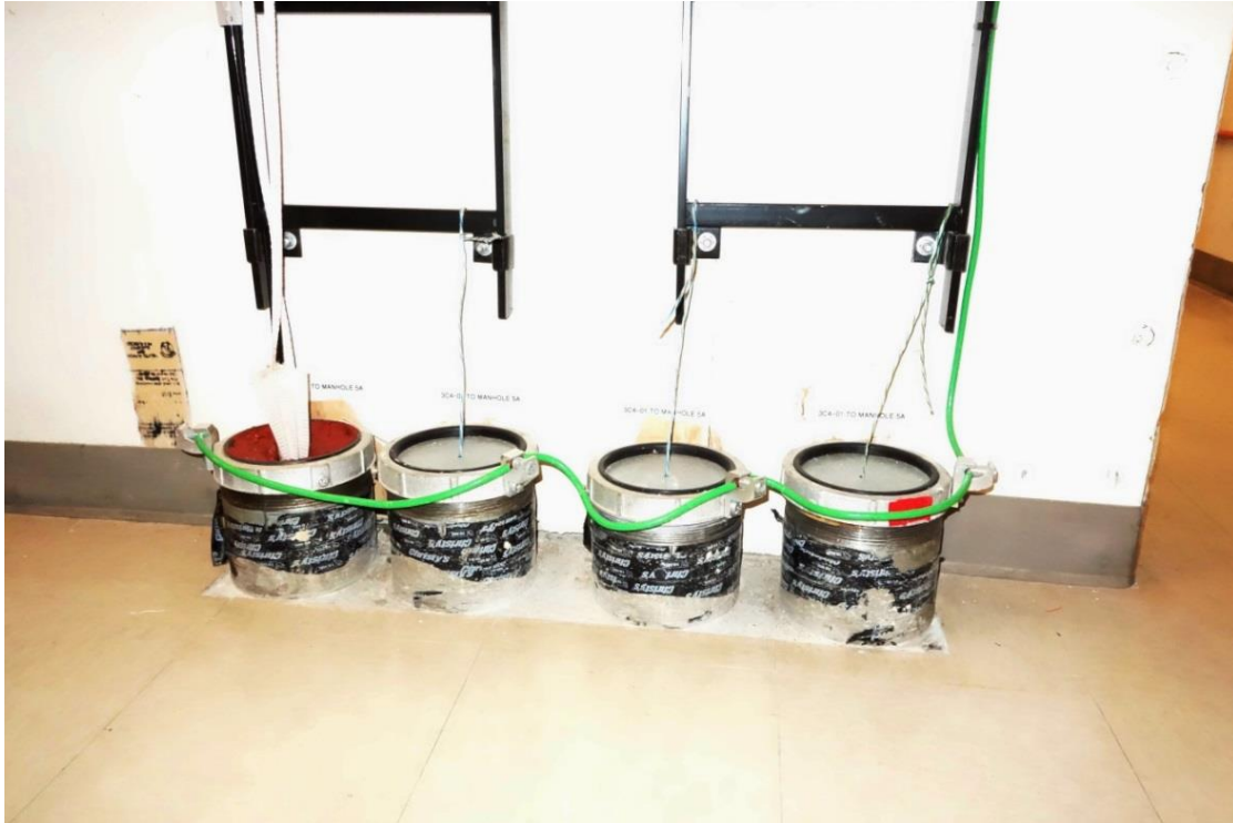
Metal conduit bushings shown with grounding wires.
