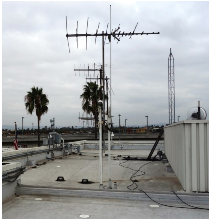
Roof-mounted antenna higher than 6-feet.
