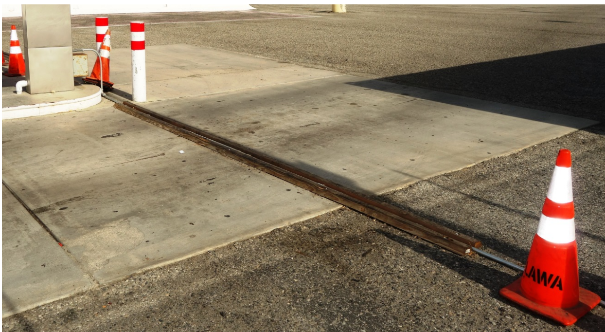
Conduit-protector at fuel pump protecting conduit.
