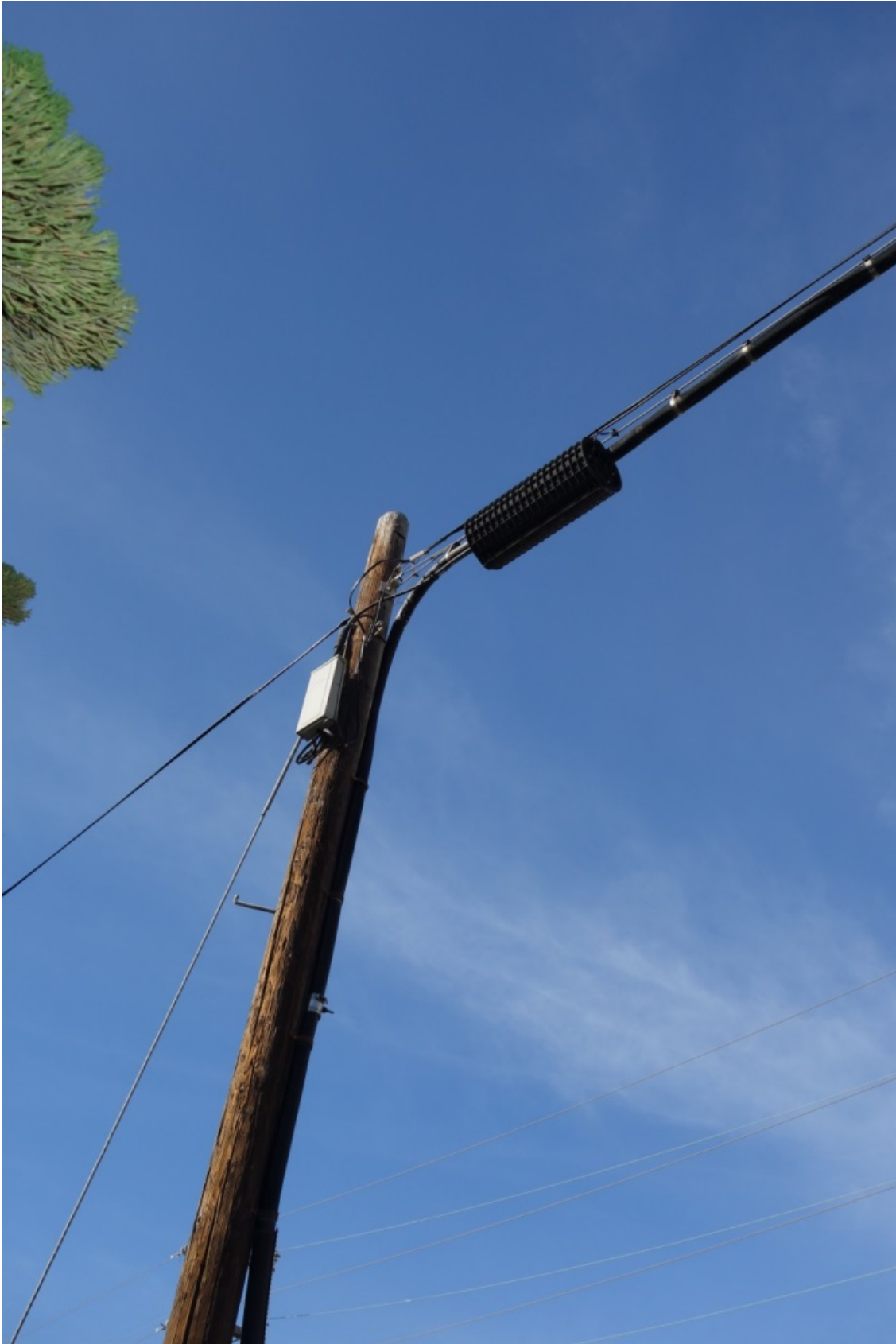
Splice case on aerial pole for comm.
