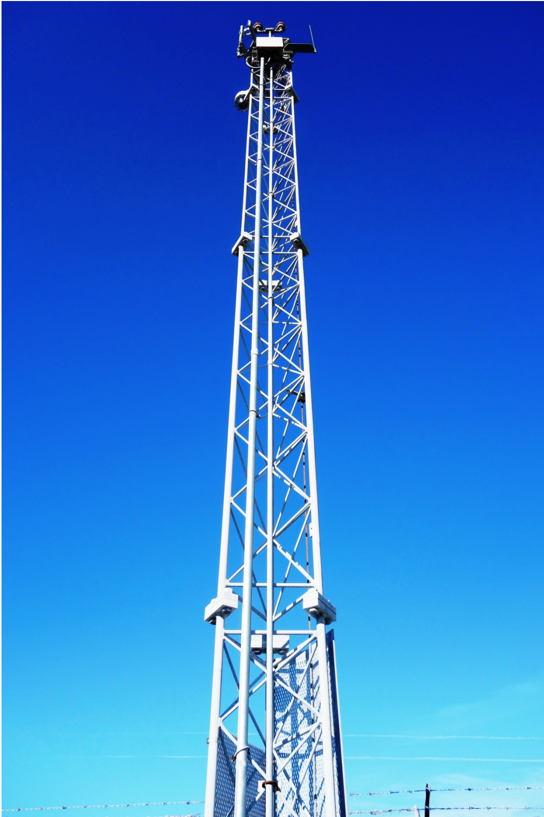
An antenna tower with two FAA-certified red flashing obstruction lights on the top.
