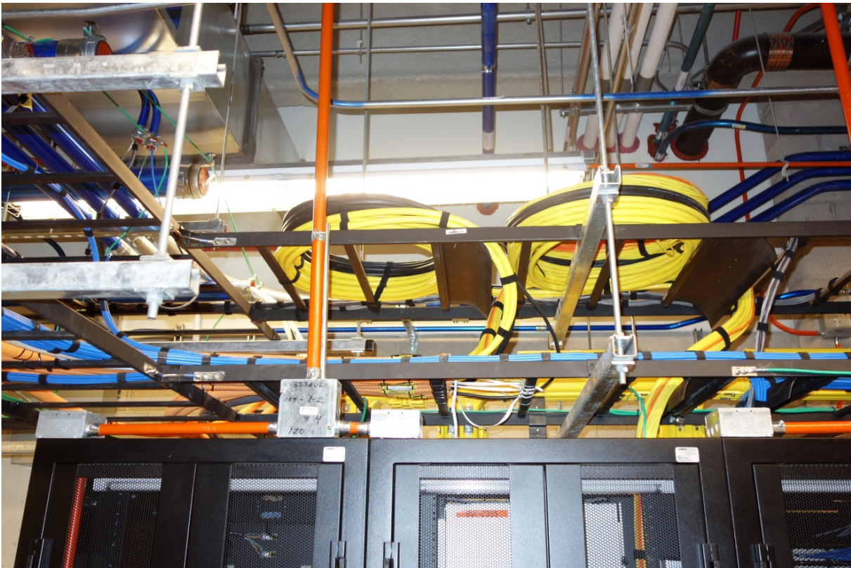
One approved method of storing cable slack loop is to build a 2 nd tier Ladder Rack.
