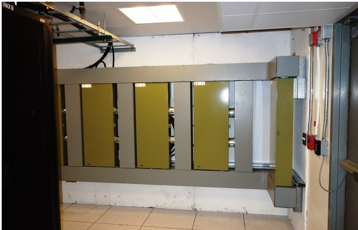
Side view of a wall-mounted fiber patch panels with interconnecting wireway and stand-offs.
