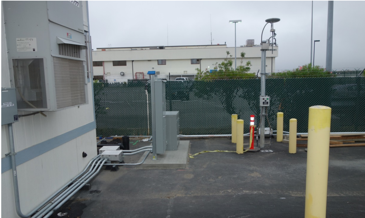
A sample of a temporary conduit installation using galvanized rigid conduit.
