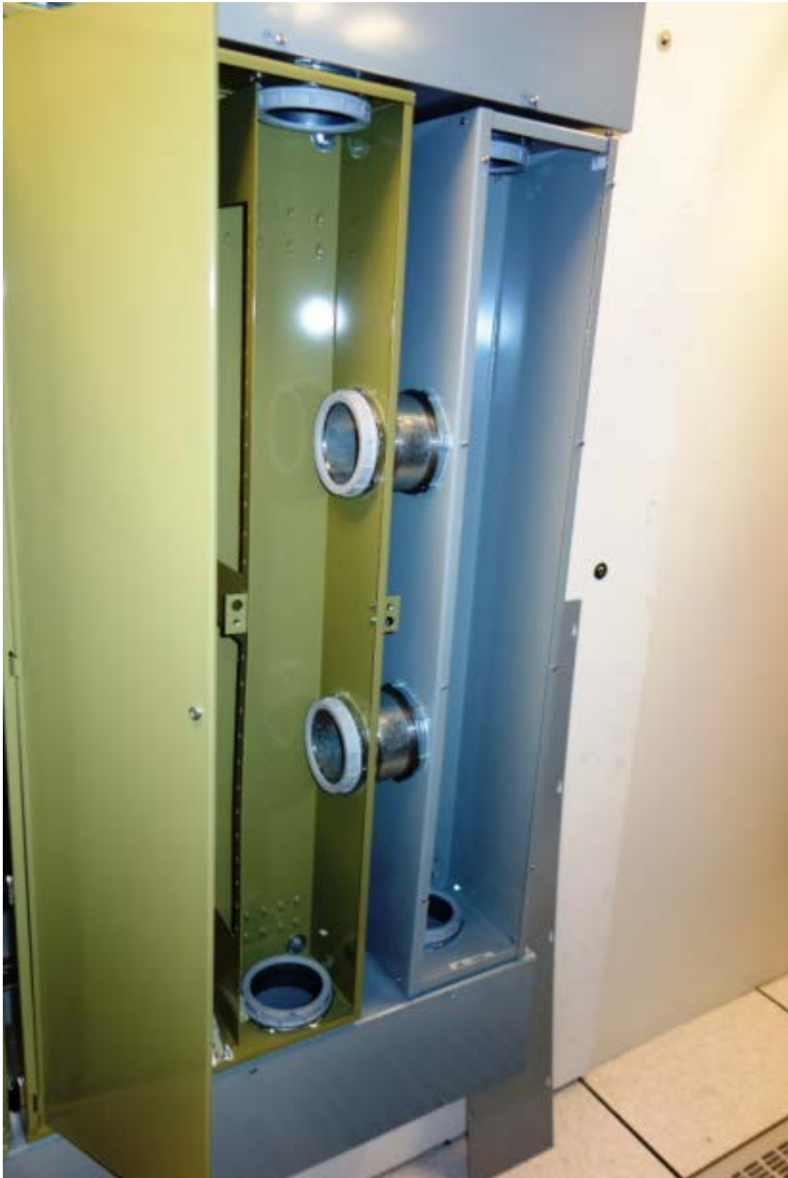
Wall-mounted fiber patch panels shall have wireway installed around and between panels.
