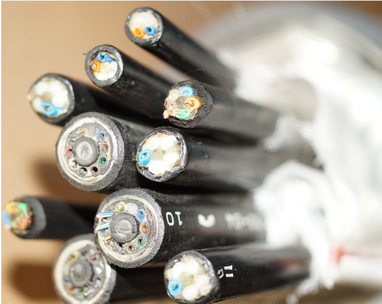
A sample of outdoor fiber cables are shown installed in a 4-inch conduit with Maxcell innerducts.
