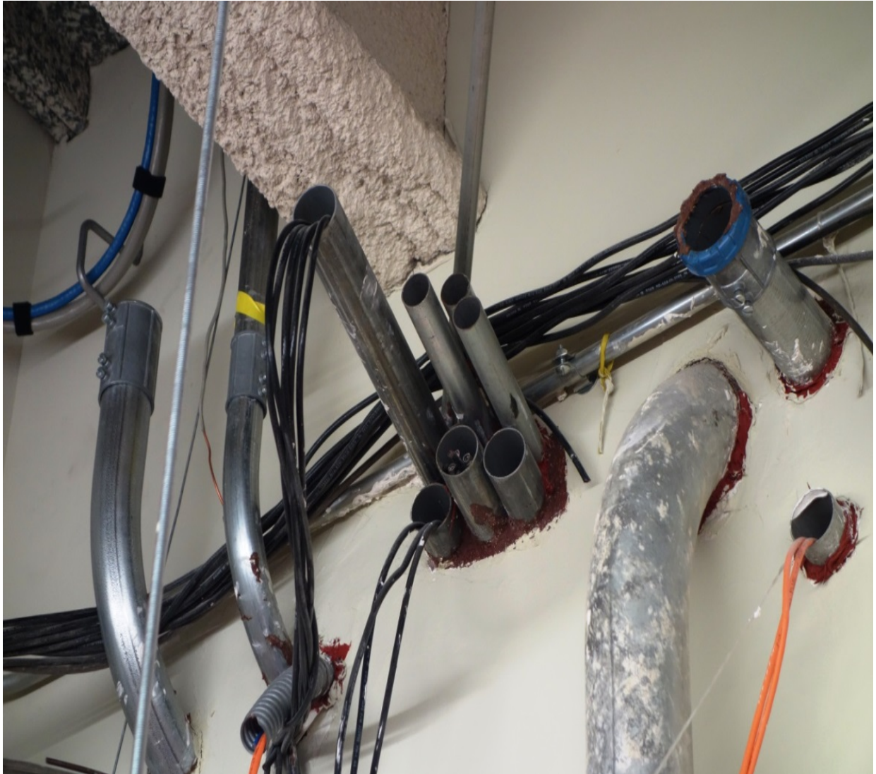
Legacy conduits are missing bushings.
