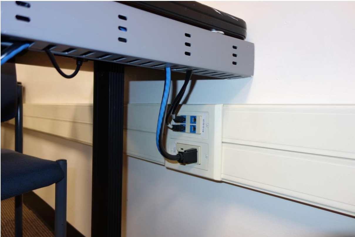
Surface-mount raceway is split to separate power and comm.
