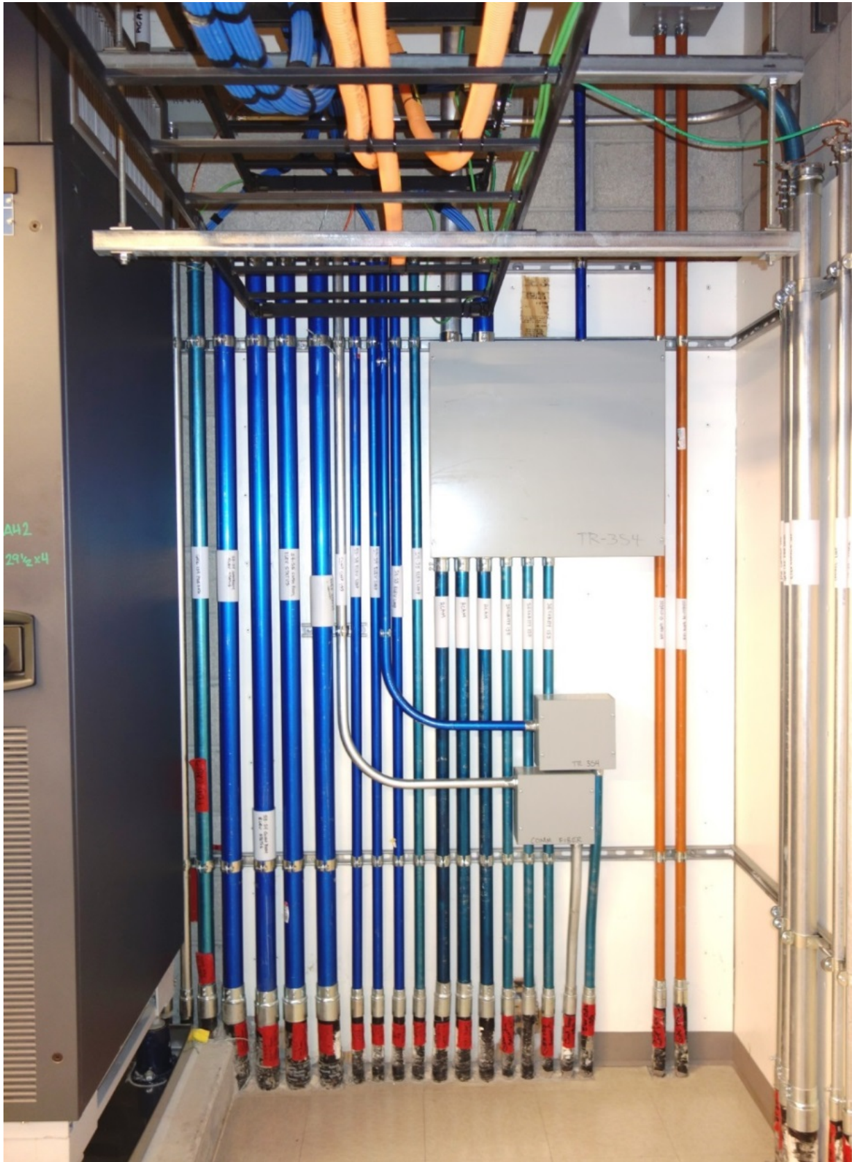
A neat, professional, blue-plated conduit installation is shown.
