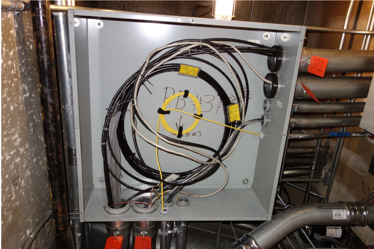
Large pull box for direction change and with slack cable loops.
