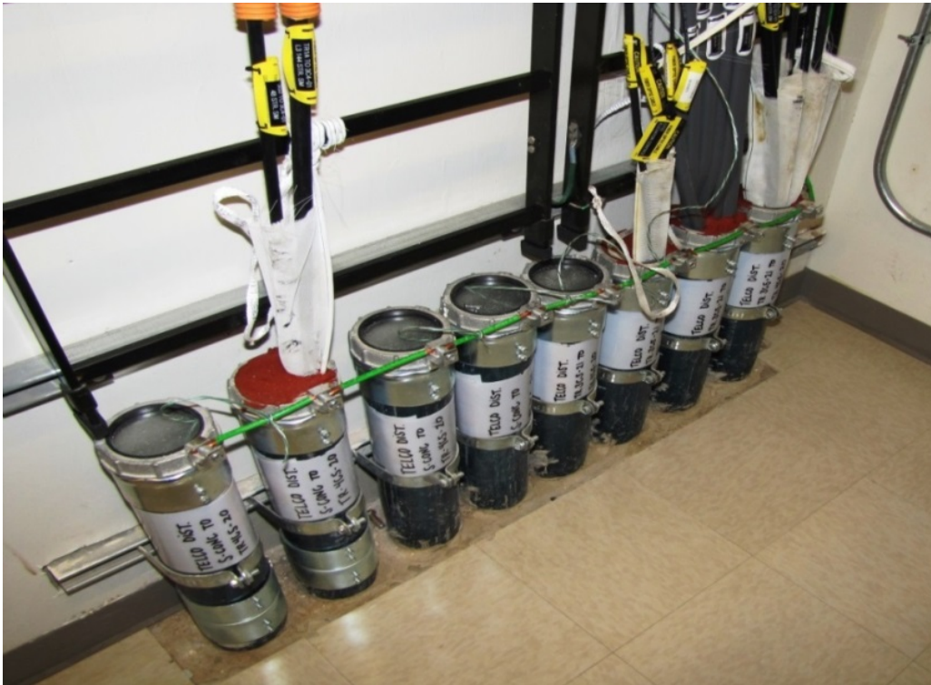
Conduit stub-ups shown secured to wall-mounted strut.
