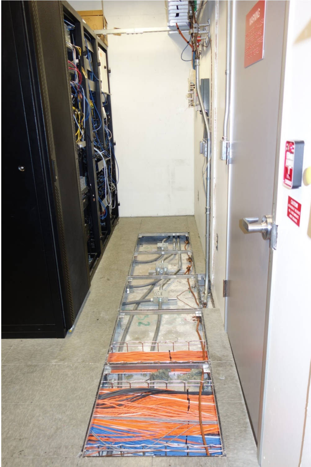
Wire basket shown running under a raised access floor for horizontal cables in an IT Room.
