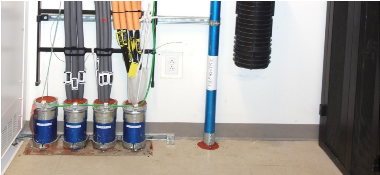
Cables routed down a wall to floor conduits shall be mounted to vertical Ladder Rack for support.
