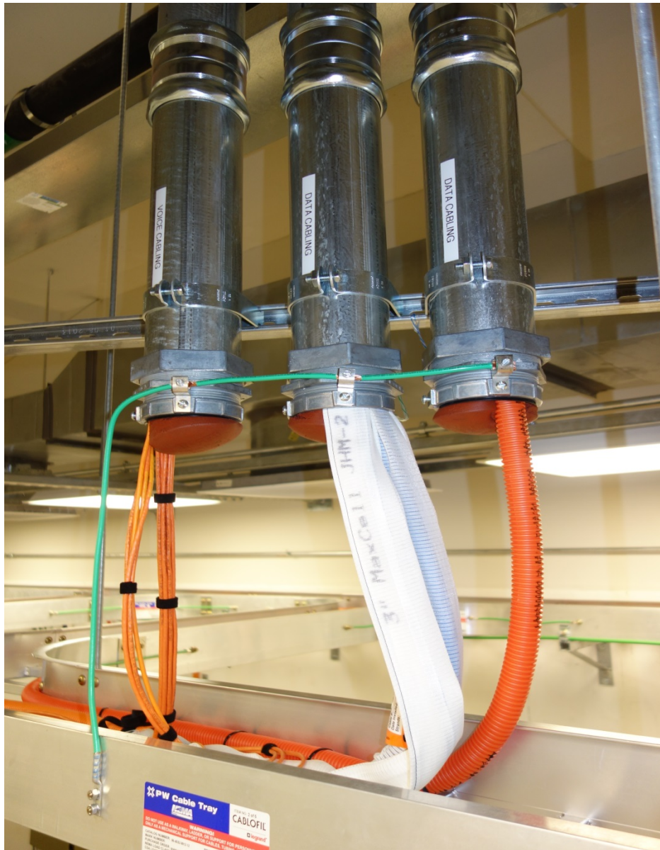
Conduits shown with HDPE innerduct that may stick inside conduit up to 6-inches.
