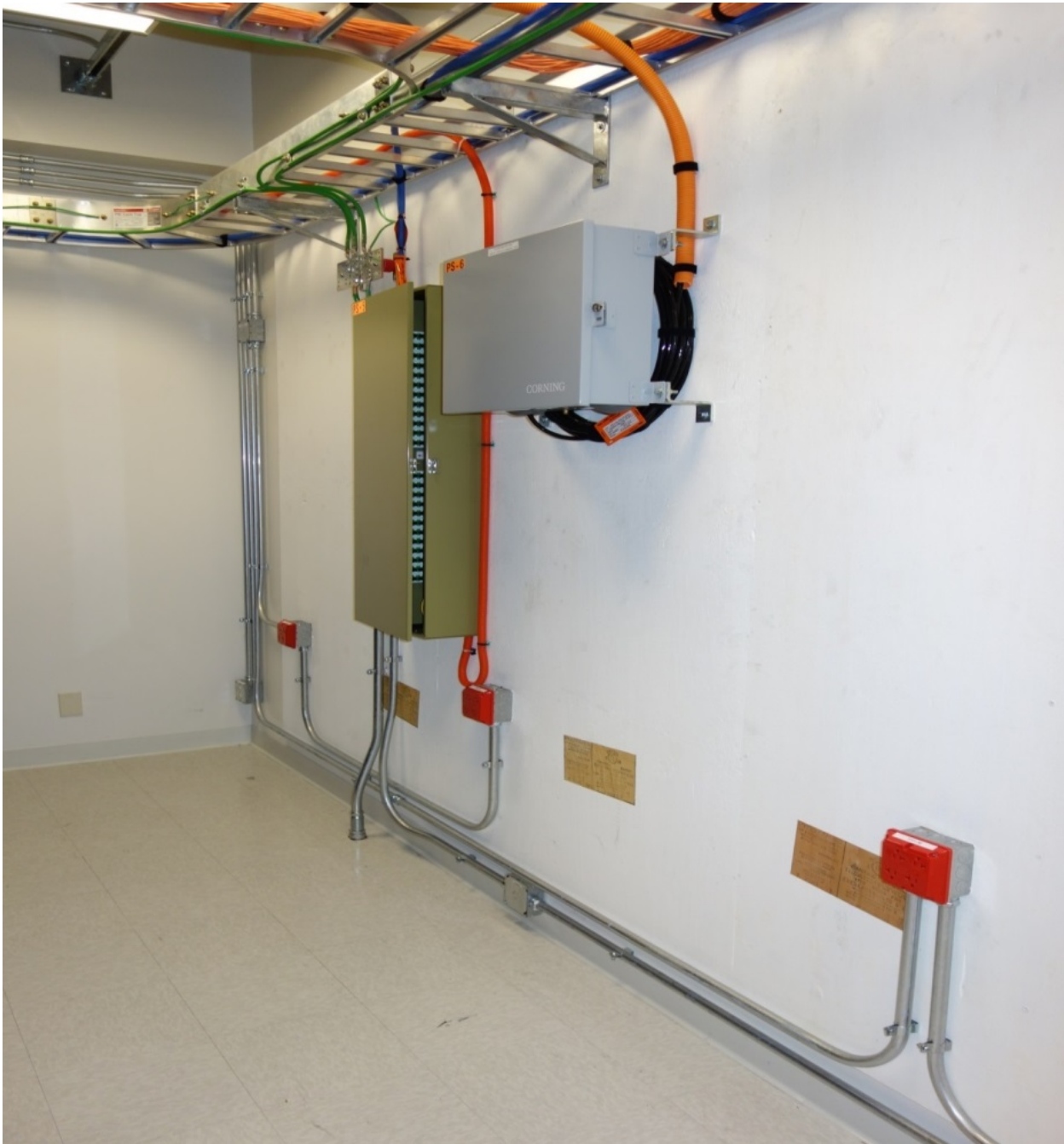
Cable slack shall be coiled up behind wall-mount patch panels.
