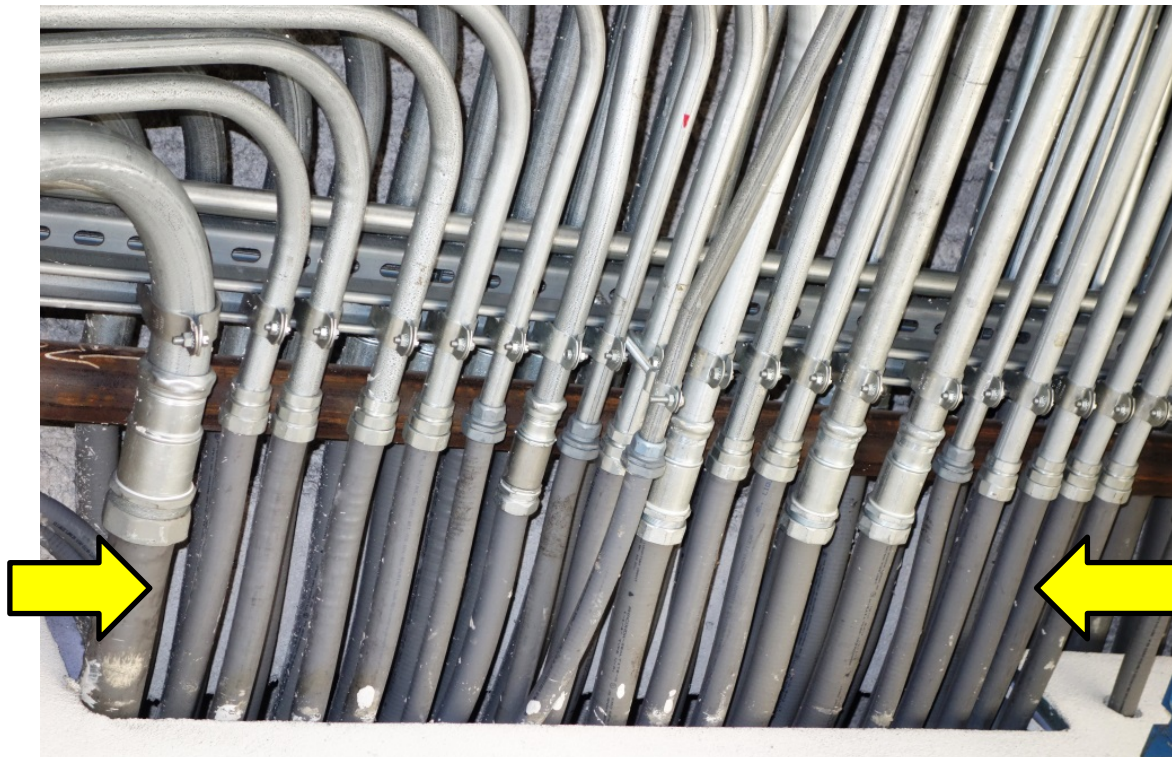
LFMC conduit expansion joints shown.
