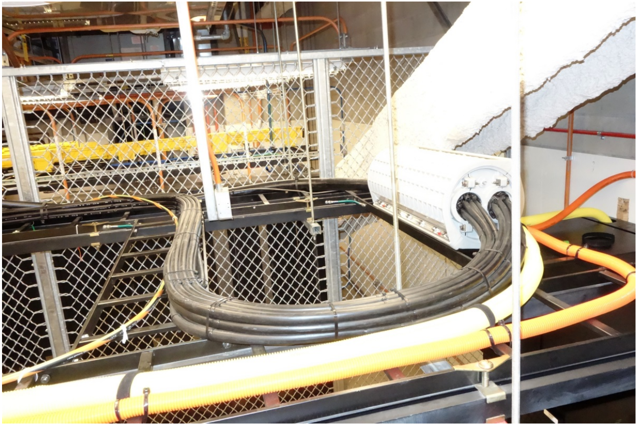
Splice case shown on a ladder rack.
