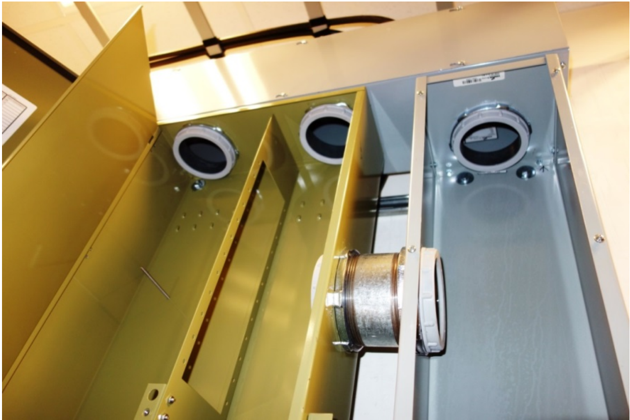
Conduit chase nipples shown connecting patch panel to top and right wireway.
