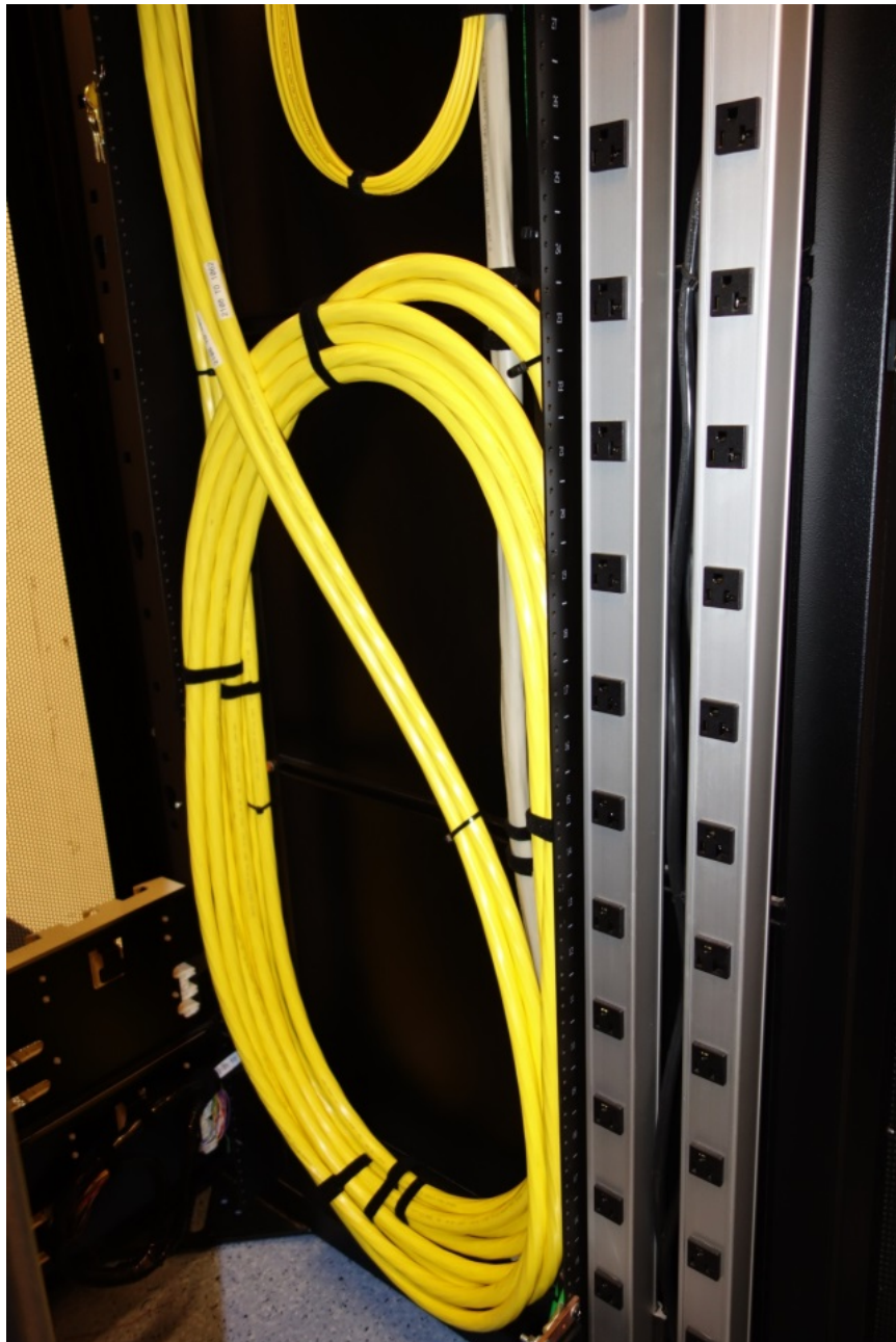
If placed within a cabinet, cable slack shall go around the inside perimeter, not coiled up.
