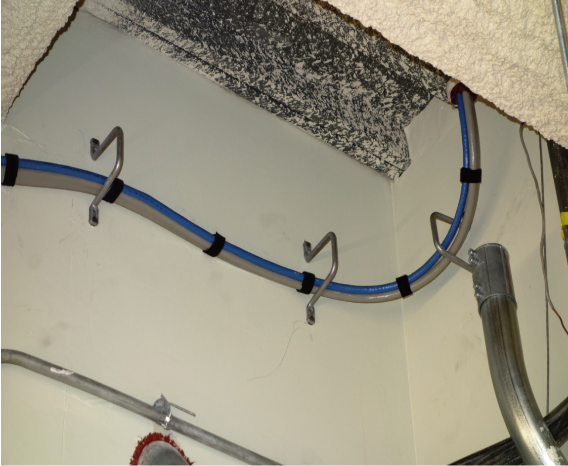
D rings used for cable management on a wall.
