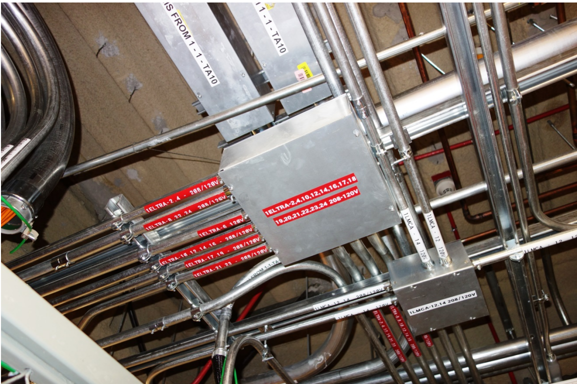
Sample pull box and conduit labeling.
