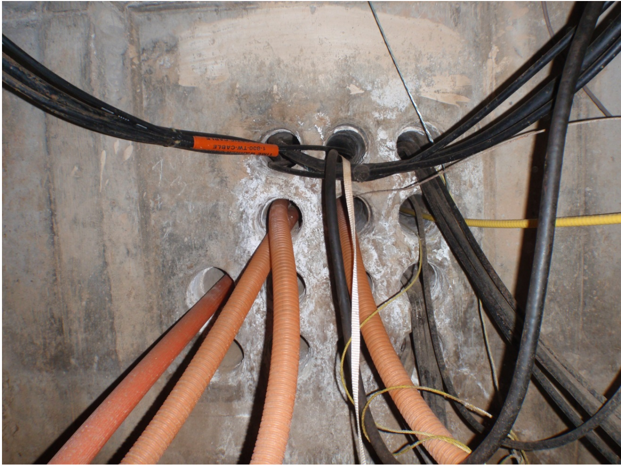
A legacy MH showing empty conduits without duct plugs and inflatable cable wraps leak.
