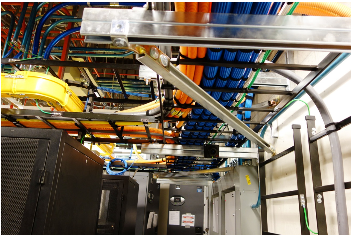
A sample ladder rack and routing install that meets LAWA's minimum requirement for a quality.
