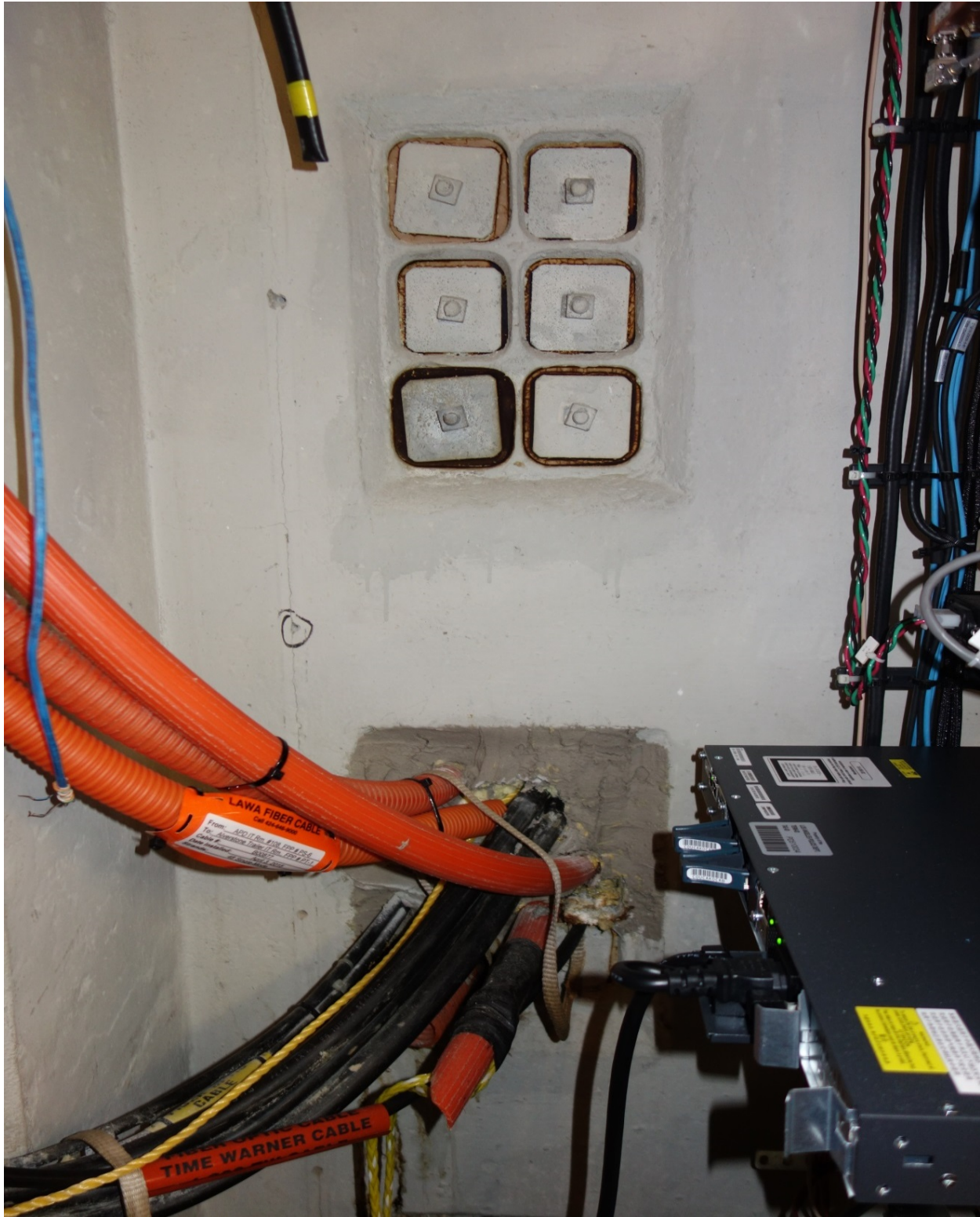
A legacy Maintenance Hole with a wall that is shared with a basement is prone to leaks.
