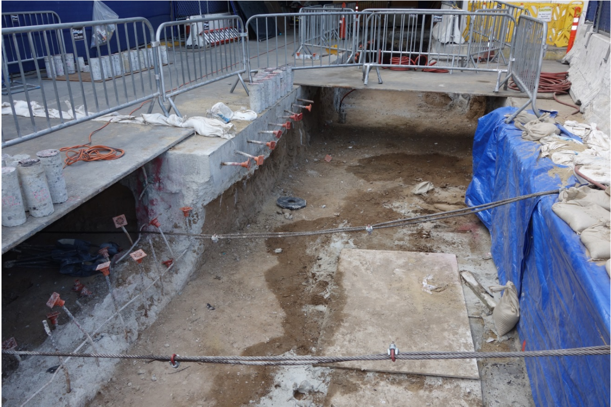
A sample excavation area awaiting fifty new 4-inch conduits where PPE is mandatory.
