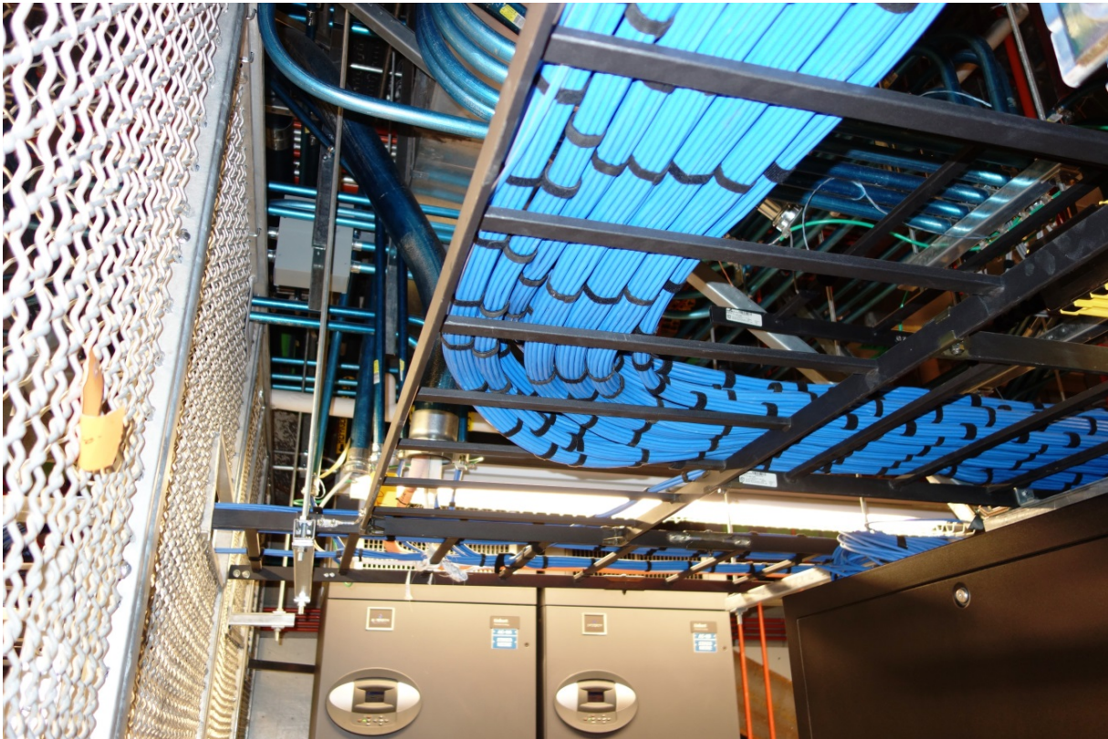
A sample horizontal cable routing that meets LAWA's minimum requirement for a quality.
