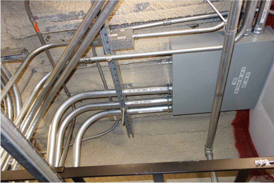
Sample pull box labeling.
