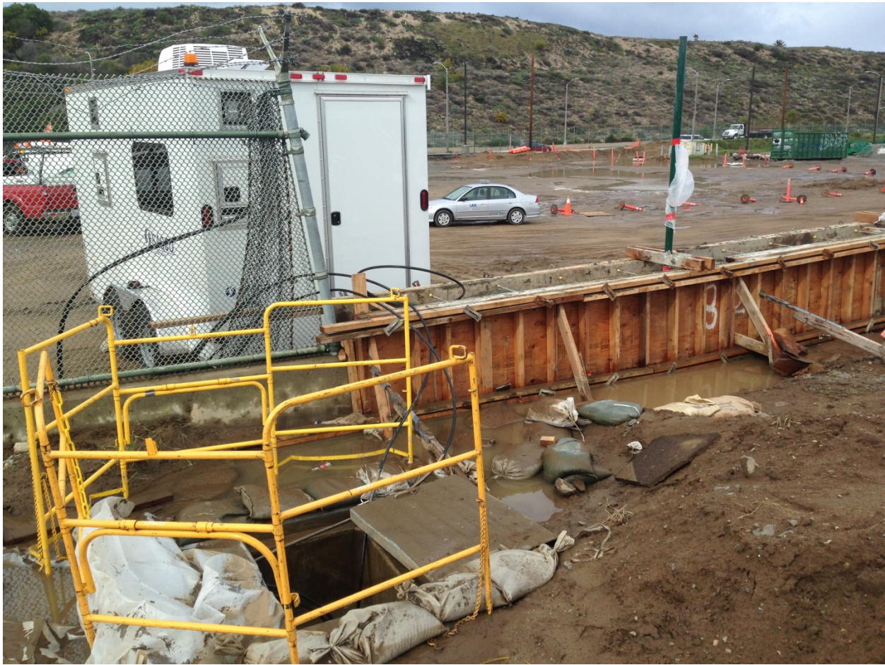
A sample of a required safety barricade surrounding a Hand Hole entrance prior to splicing.
