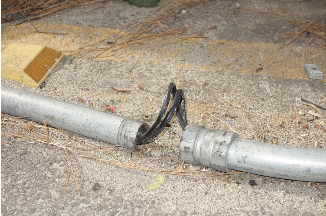
A sample of a rigid conduit coupling that has opened due to a lack of protection.
