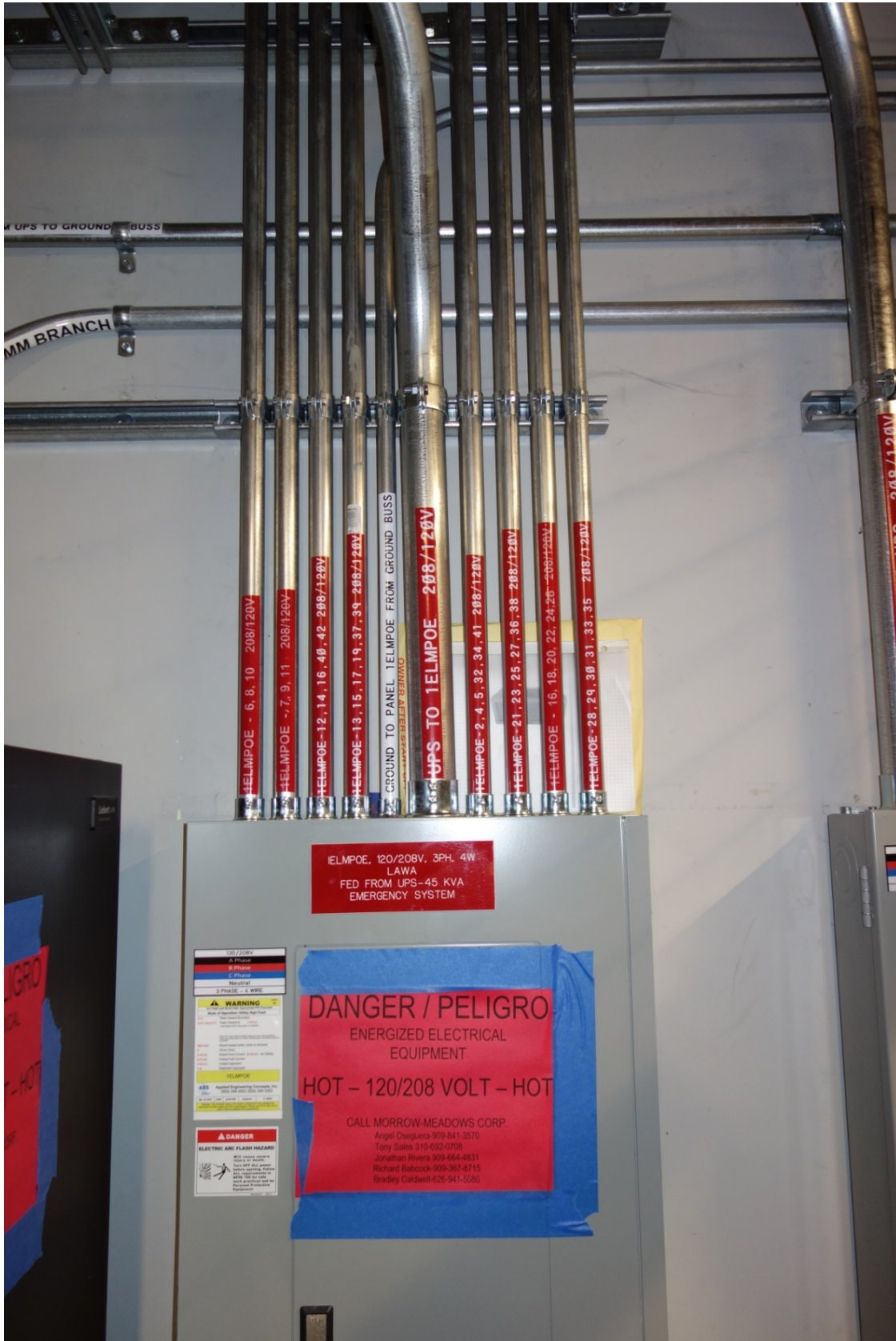
Sample electrical conduit and panel labeling.
