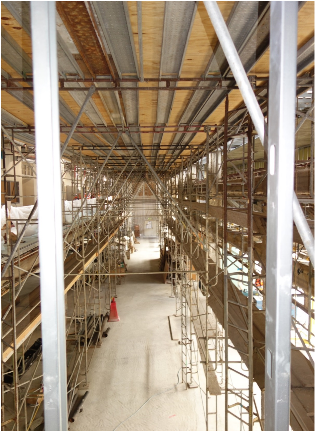
A sample terminal renovation area where PPE and extreme caution is required.
