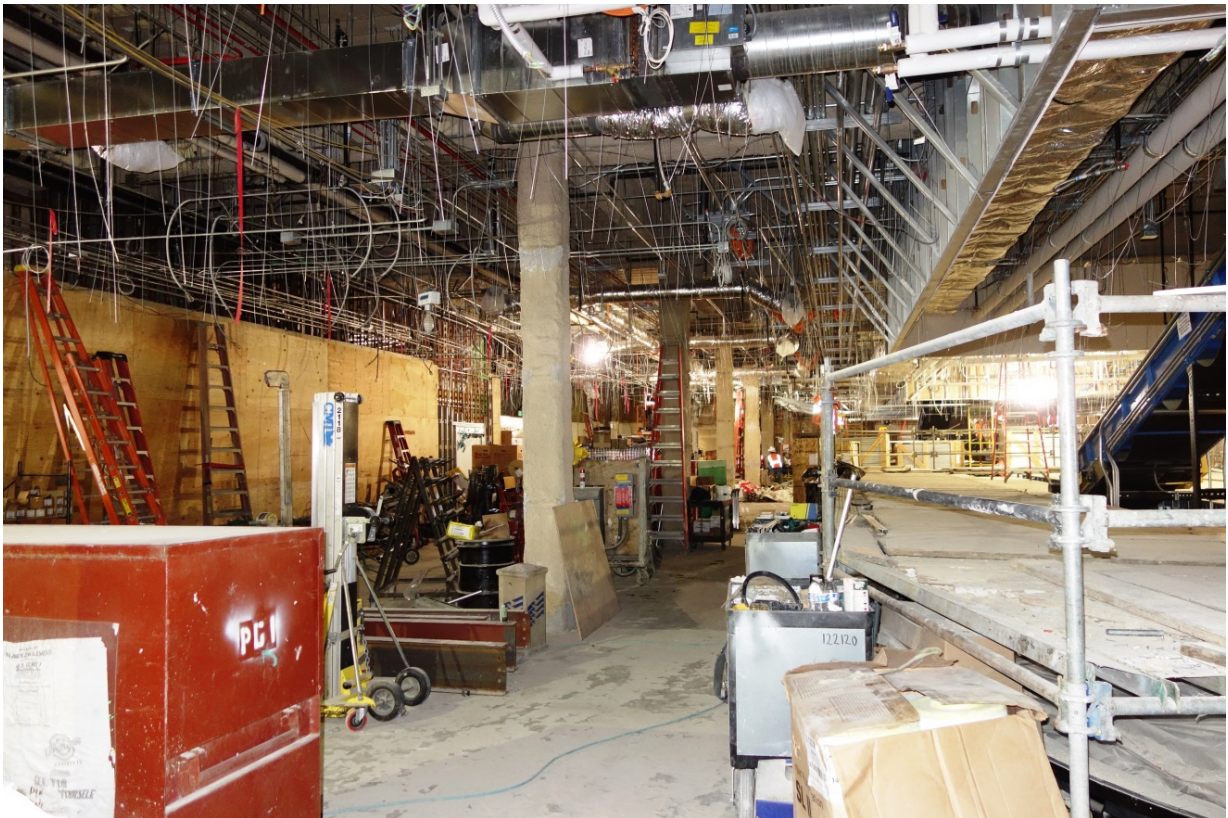
A sample terminal baggage carousel renovation area where PPE and caution is required.
