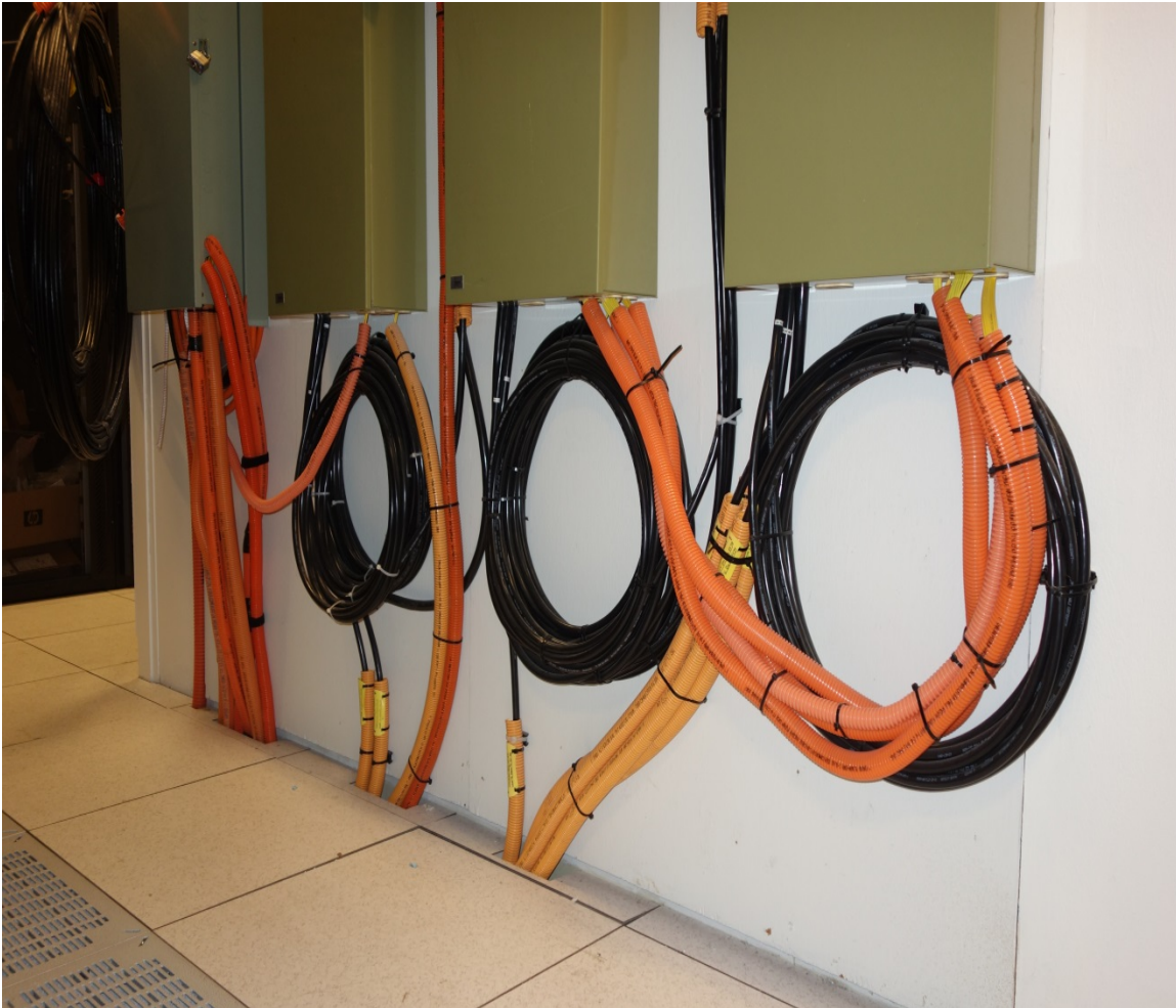
Legacy fiber slack previously mounted on walls is not coiled up behind patch panels.
