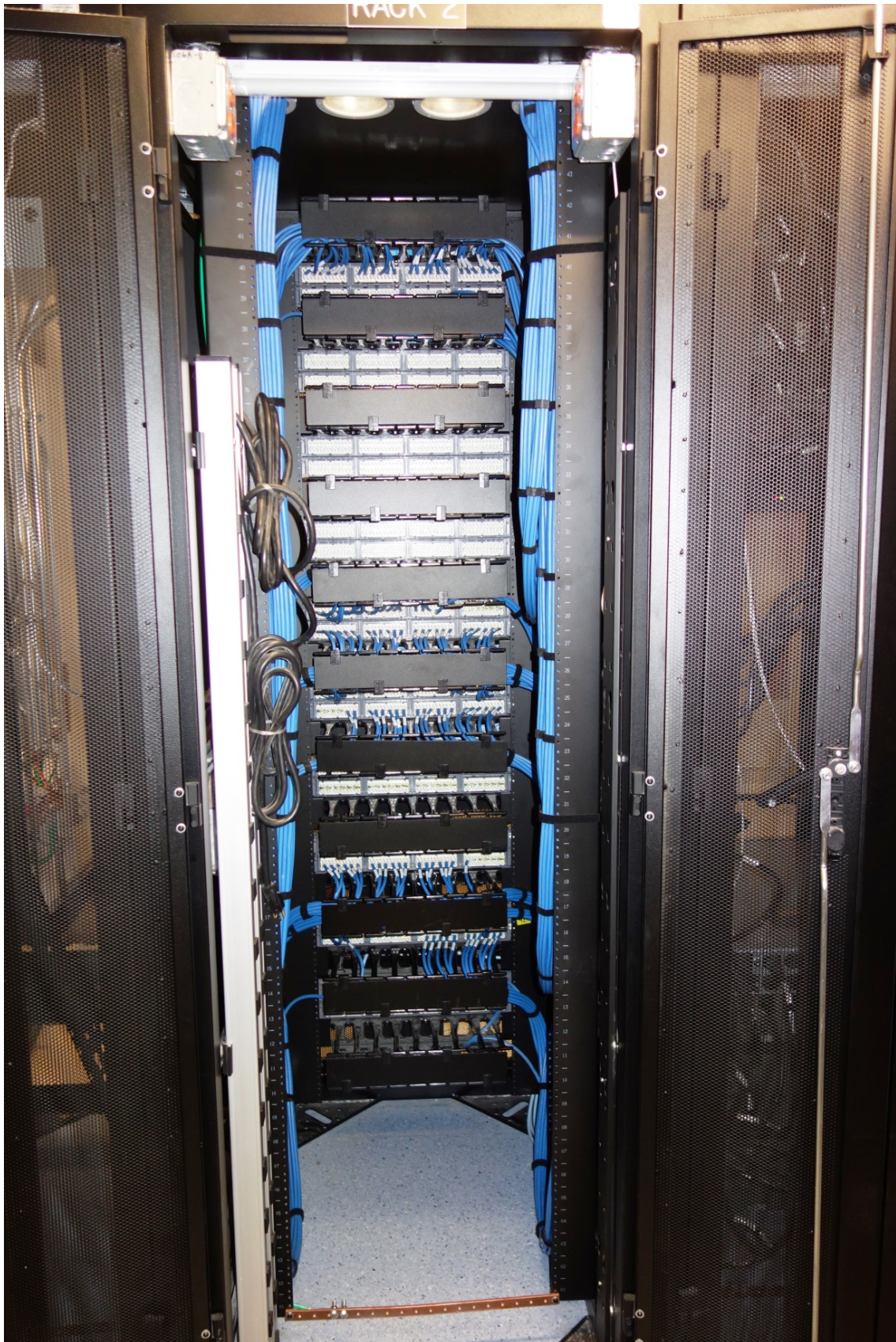
A sample CAT 6A cable installation that meets LAWA's minimum requirement for a quality.
