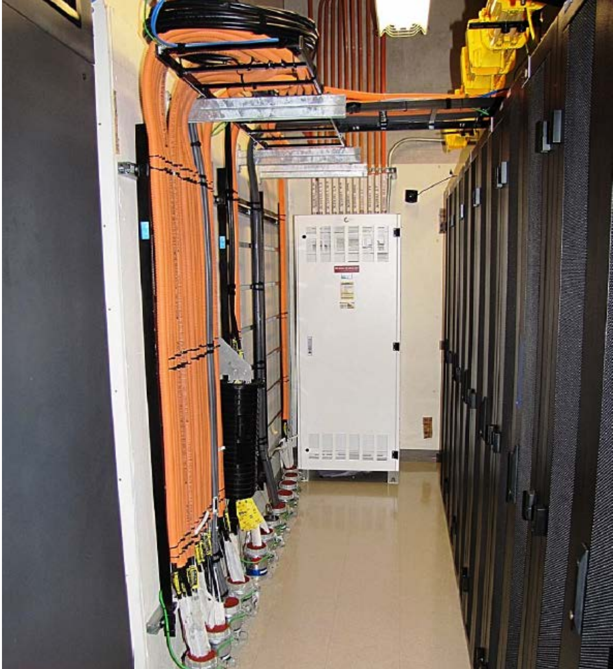
A sample IT Room that meets LAWA's minimum requirement for a quality installation.
